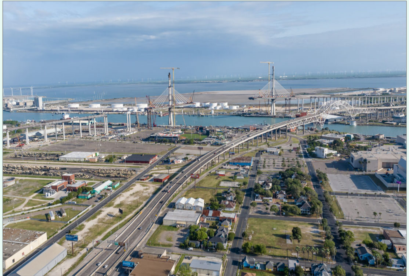
Existing Harbor Bay Bridge (foreground) and ongoing construction of the new Harbor Bay Bridge which will open Spring 2025
