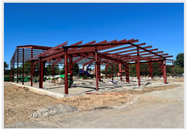
Bottom Right: a view of the overall progress at the Yahara Site of the new Maintenance Building as the steel structure is erected
