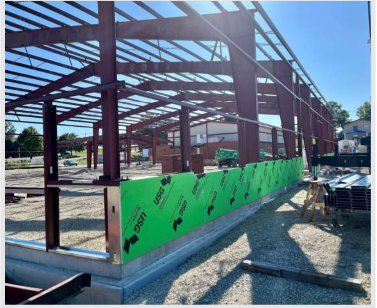
Top Right: a look at the progress at the Maintenance Building as exterior framing and sheathing goes into place
