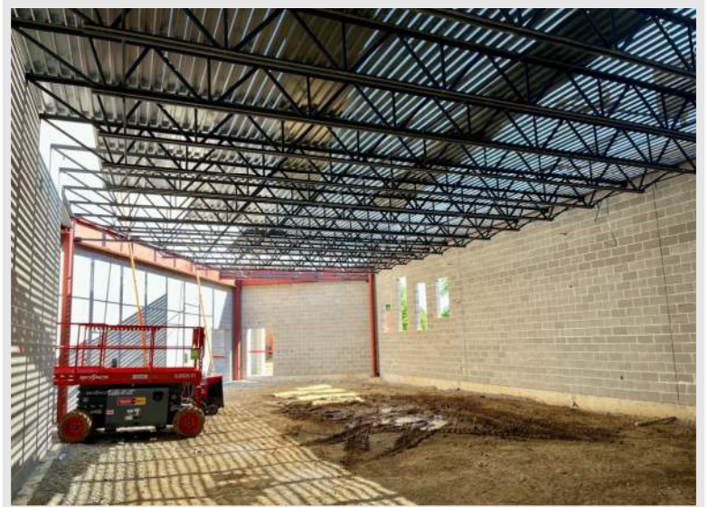
Above: a view of the future Athletics Room as metal decking is installed atop the steel joists overhead
