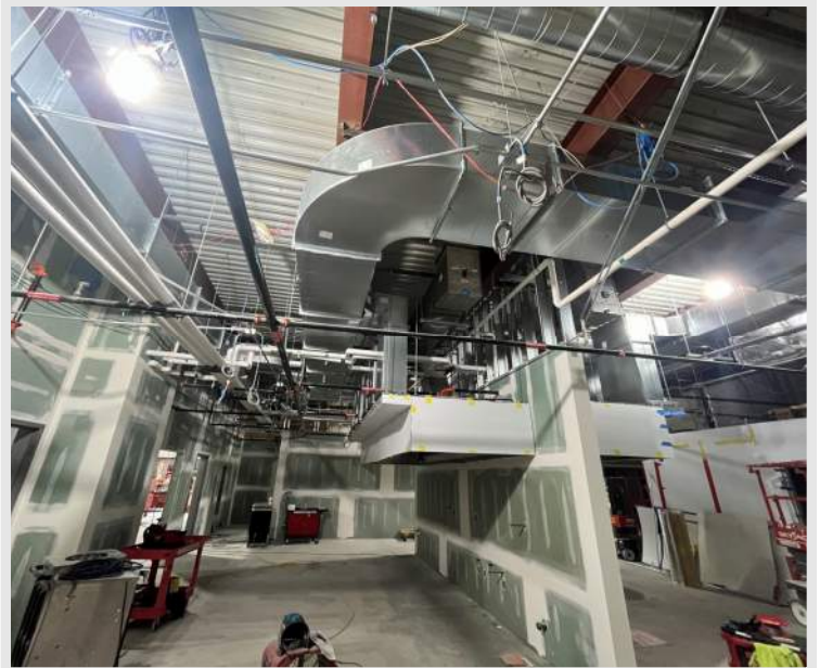
Bottom Right: a look at the progress in the High School kitchen of drywall tape & finish with MEP rough-ins overhead
