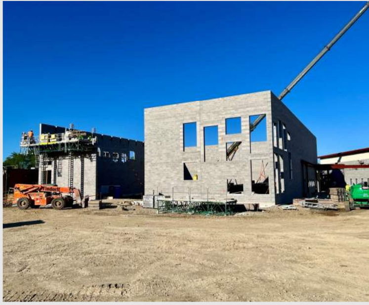
Top Left: a view of the sun shining down on the River Bluff addition as the final CMU walls are set
