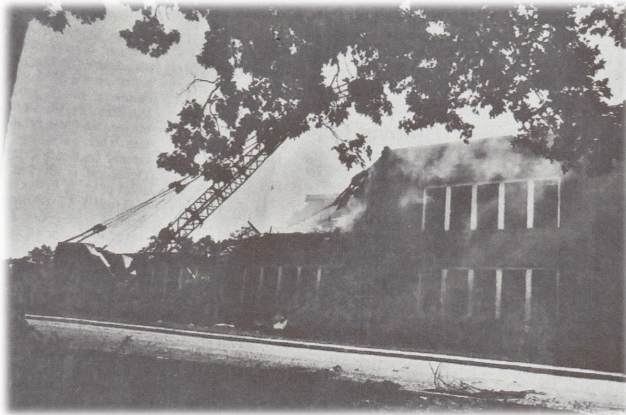
July 8, 1982 Demolition of Star Middle School for new Star-Biscoe Elementary School building.
