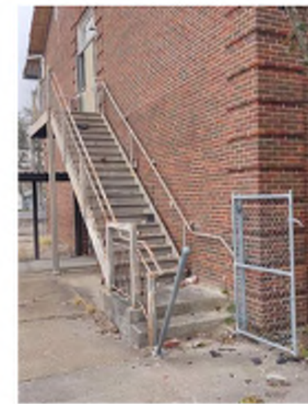
7C. SOUTH STAIR - NON-COMPLIANT GATE
