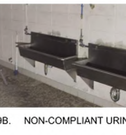
9B. NON-COMPLIANT URINALS
