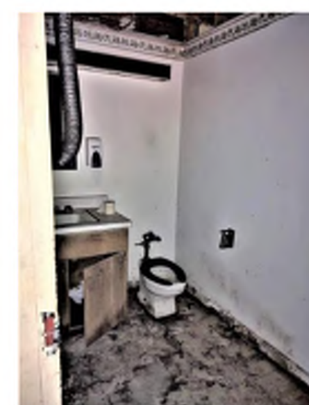
9C. NON-COMPLIANT STAFF RESTROOM
