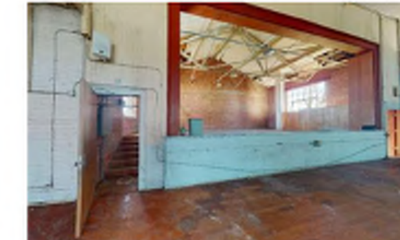
11A. NON-ACCESSIBLE STAGE - LEFT ENTRANCE
