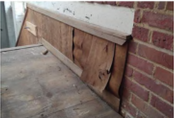
5D - DAMAGED WOOD PANELING
