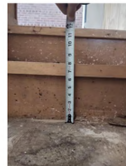
8B. EAST INTERIOR STAIR - NON-COMPLIANT TREAD
