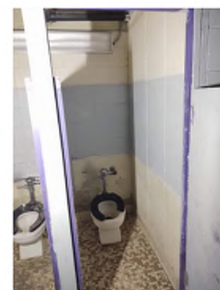
9B. NON-COMPLIANT STALLS
