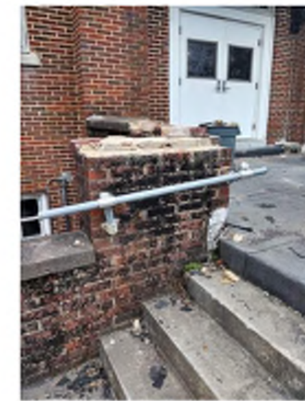
7D. WEST STAIR - NON-COMPLIANT RAIL
