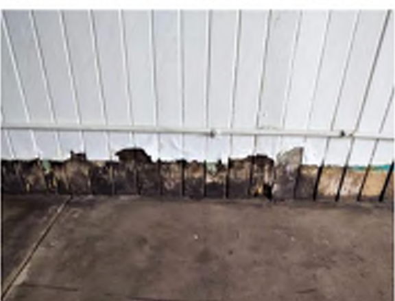
5F - DAMAGED WOOD WAINSCOT
