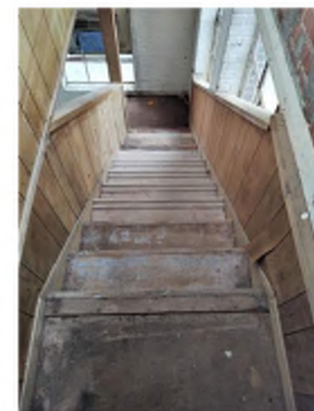
8A. EAST INTERIOR STAIR - NON-COMPLIANT RAIL
