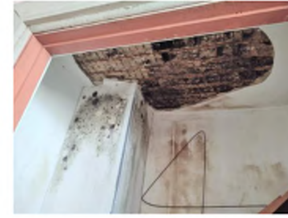
5A - COLLAPSING PLASTER CEILING
