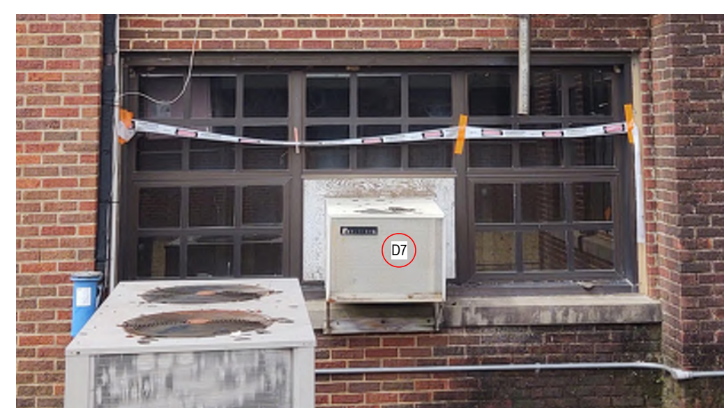
13 ALUMINUM WINDOW AT AC UNIT
