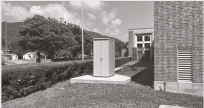
A new generator was installed at the MS/HS.
