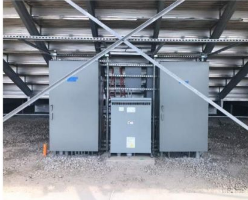
6.11.24 - Main Distribution Panel and Transformer at Home Grandstands
