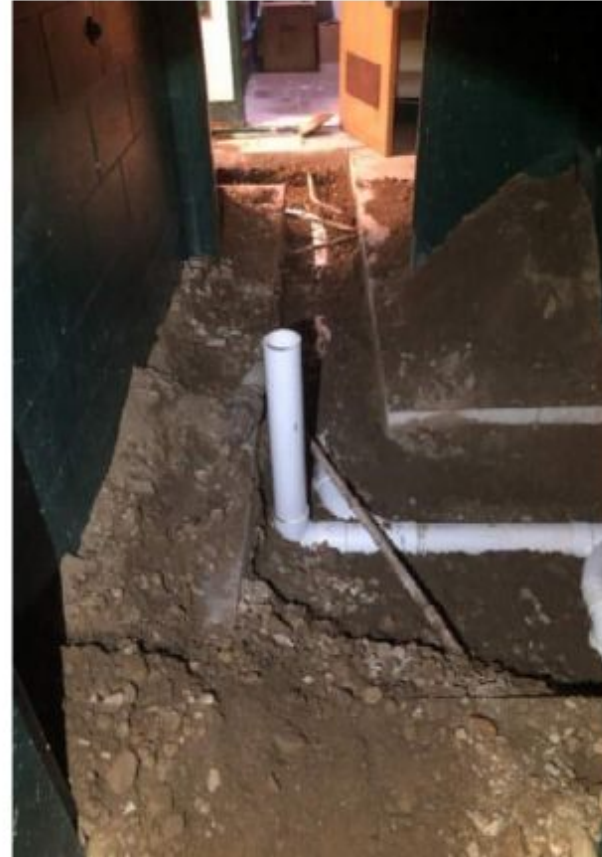
6.12.24 - MS Plumbing Repairs - New Underground Sanitary Line at Area 1 - Boys Locker Room
