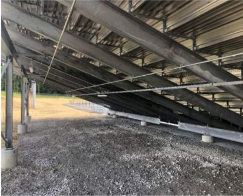
6.11.24 - Electrical Conduit and Lights at Visitor Grandstands
