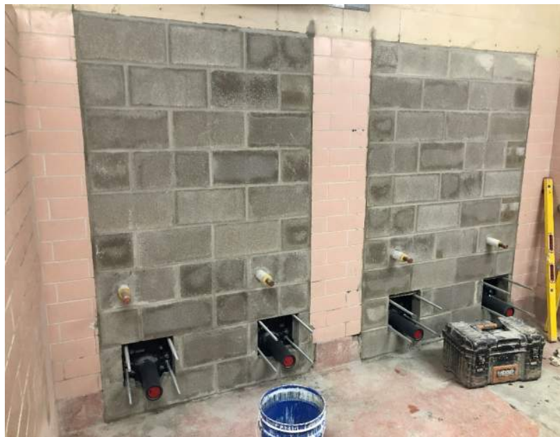
7.9.24 - Girl's Group Restroom, Masonry infil
