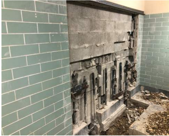
6.12.24 - Middle School Plumbing Repairs - Floor and Wall Demolition at Area 4 - Boys Group Restroom
