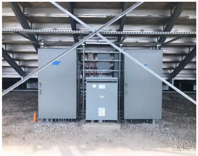
6.11.24 - Main Distribution Panel and Transformer at Home Grandstands
