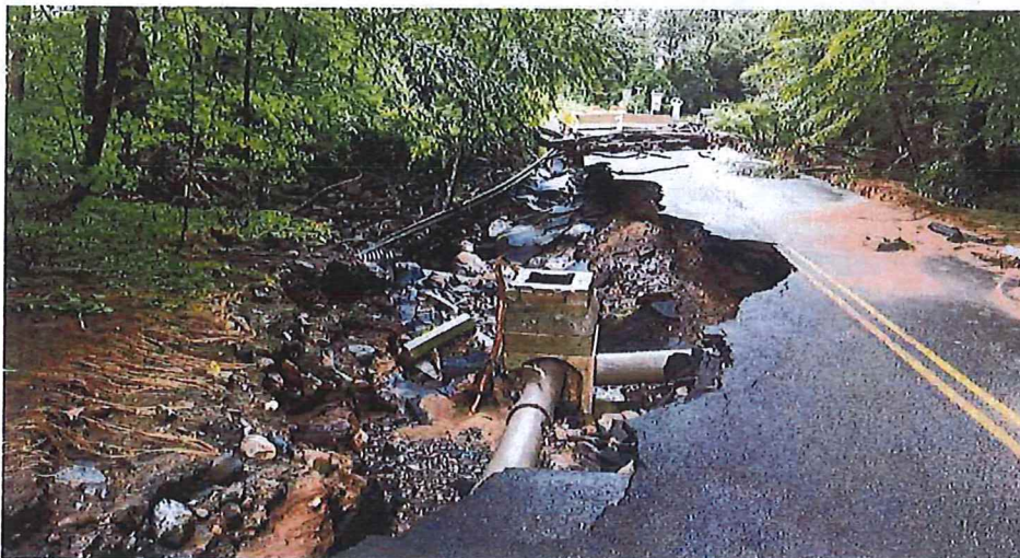
A section of washed-out road on Cottage Street in Monroe on Monday.
