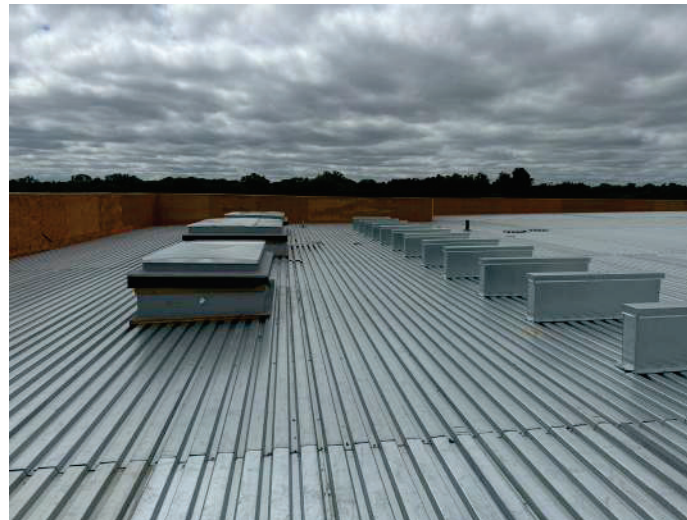
RTU and Condensing Unit Curbs
