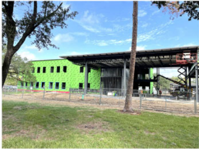
Two story Academic Wing on the left in green sheathing and library steel framing on the right
