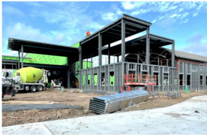
View from parents drive toward main entry. Repurposed library into new administration area on the right.
