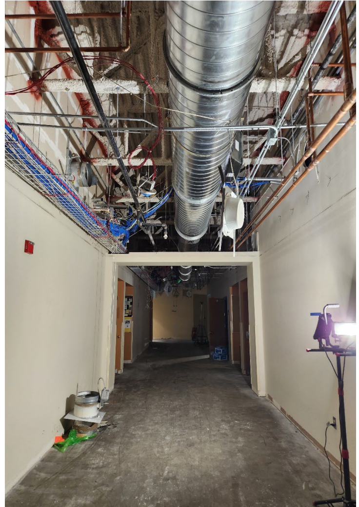
LOHS Science Hallway New Larger Ductwork
