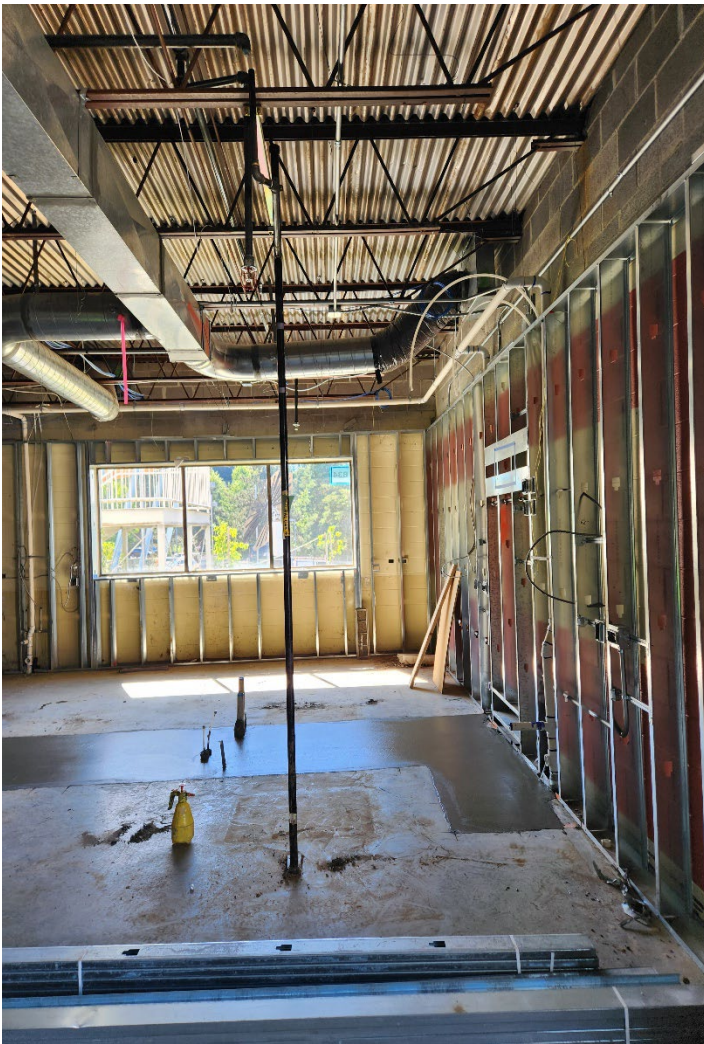
LHS Science Classroom MEP
