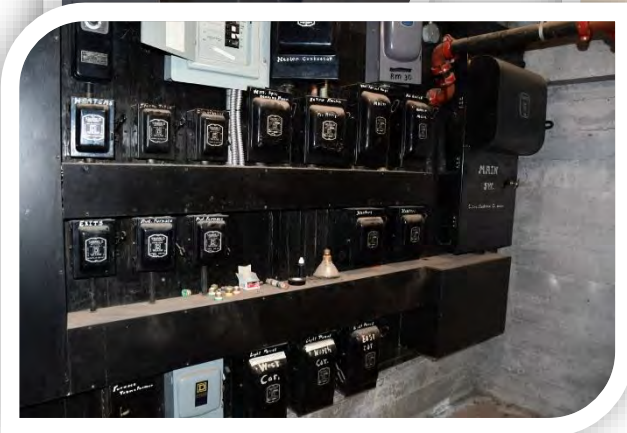
Outdated electrical systems
