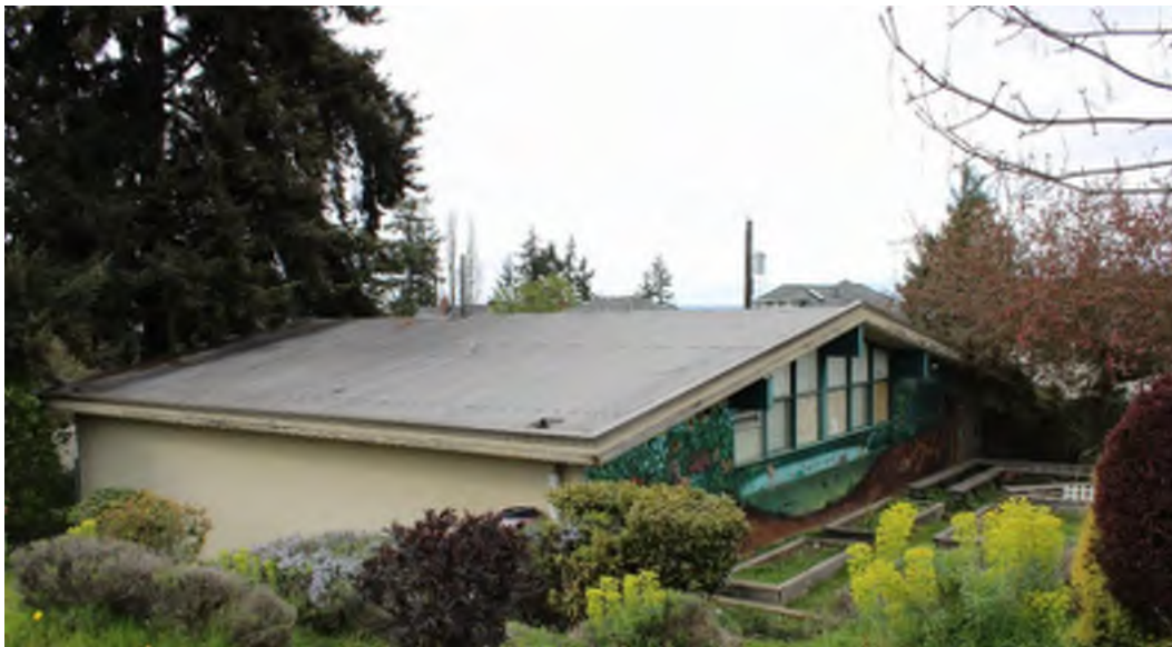
Figure 28: A portion of the quad structure that makes up the Lowell ES annex. View to the SE.
