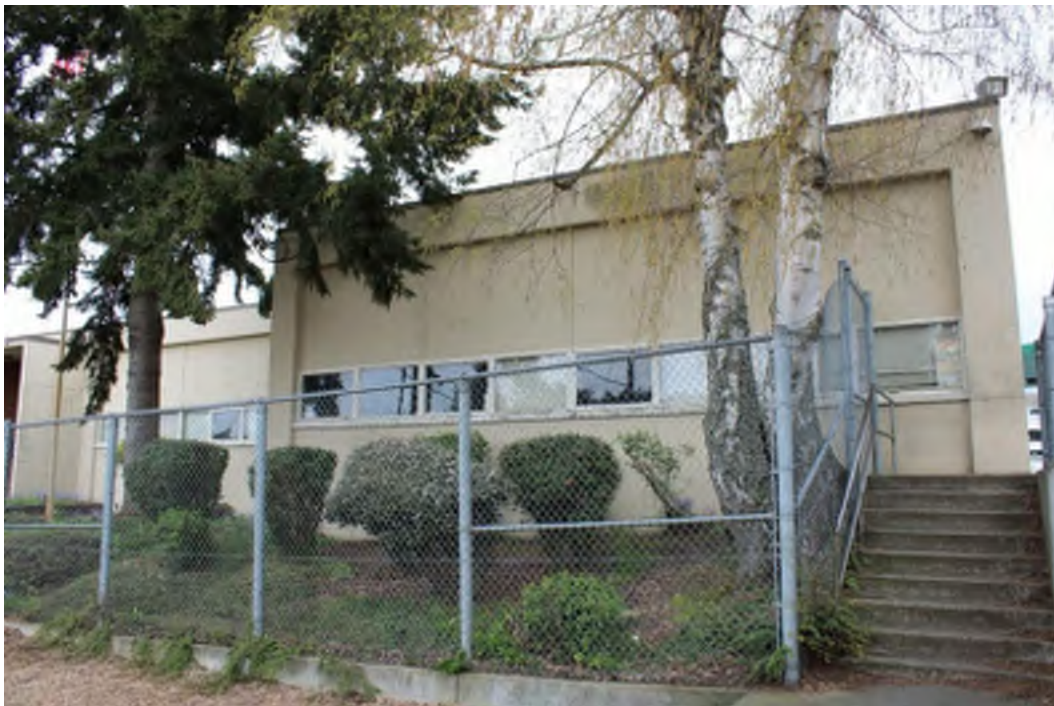
Figure 26: A portion of the north façade near the main entrance. View to the south.
