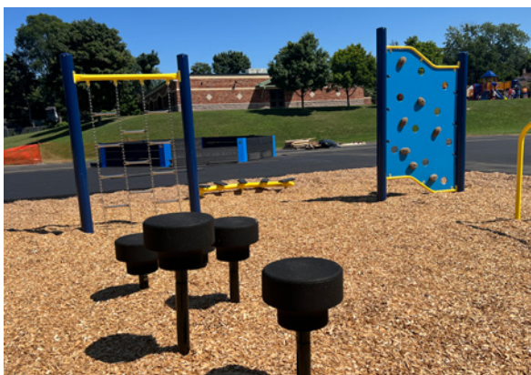
Construction on new playgrounds at Iroquois and Rogers middle schools was completed in August. They each include two popular Gaga Ball pits, as well as more traditional equipment for grades 4-6 students to use.
