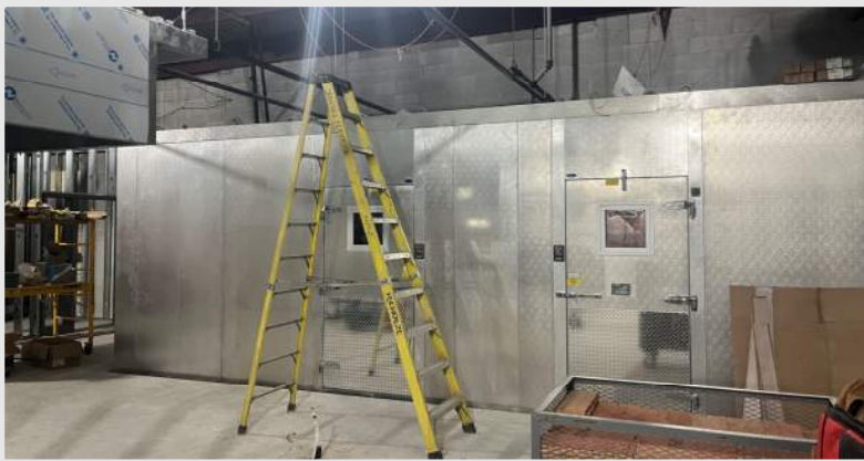
Top Left: a photo of the new cooler & freezer installed in the High School kitchen
