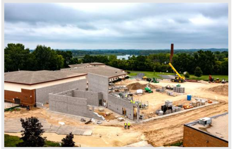
Above: a view of the overall progress at the River Bluff Middle School addition captured by a Findorff drone flight on 8/5
