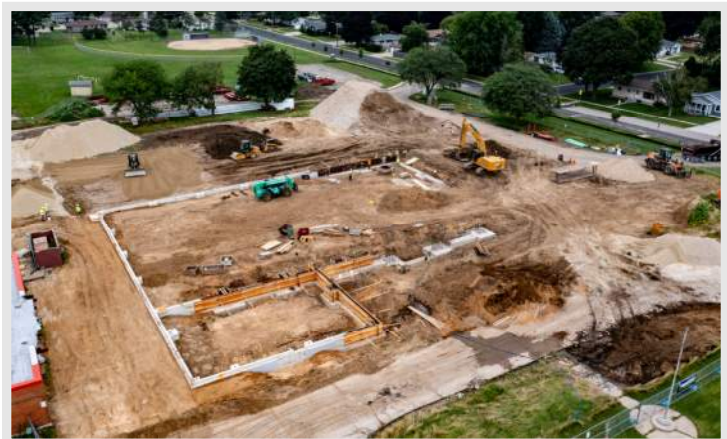
Above: a photo captured from a Findorff drone flight on 8/5 highlighting the progress on foundations for the Maintenance Building
