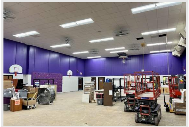
Above: a sneak peak of the new finishes in the Kegonsa Elementary Gym / Cafeteria space ahead of the flooring install
