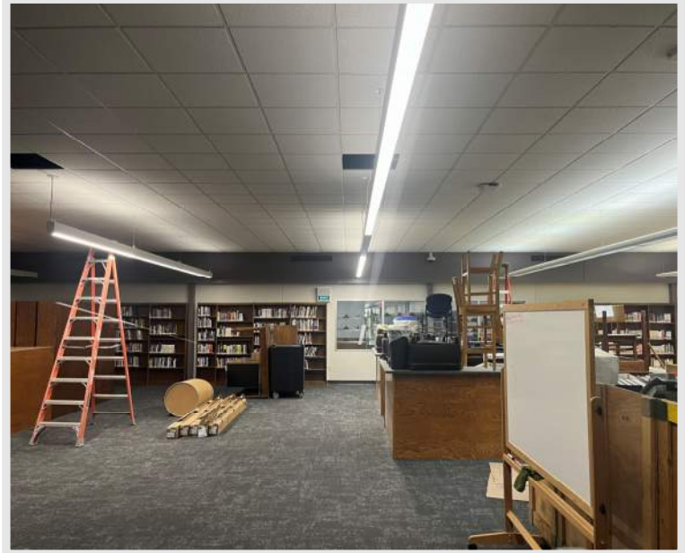
Top Right: a view of the new light fixtures and ceiling installed in the High School library
