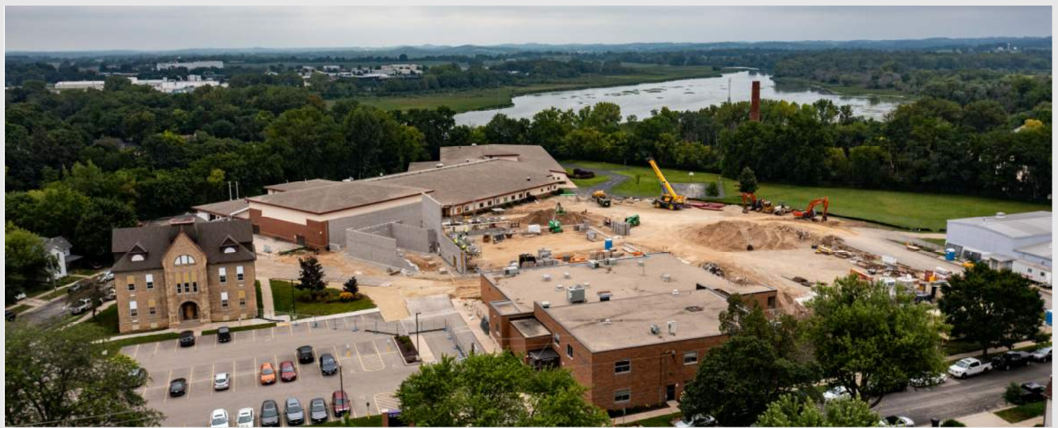
Bottom: a photo captured of the River Bluff Campus highlighting the over progress in the foreground and Yahara River in the background
