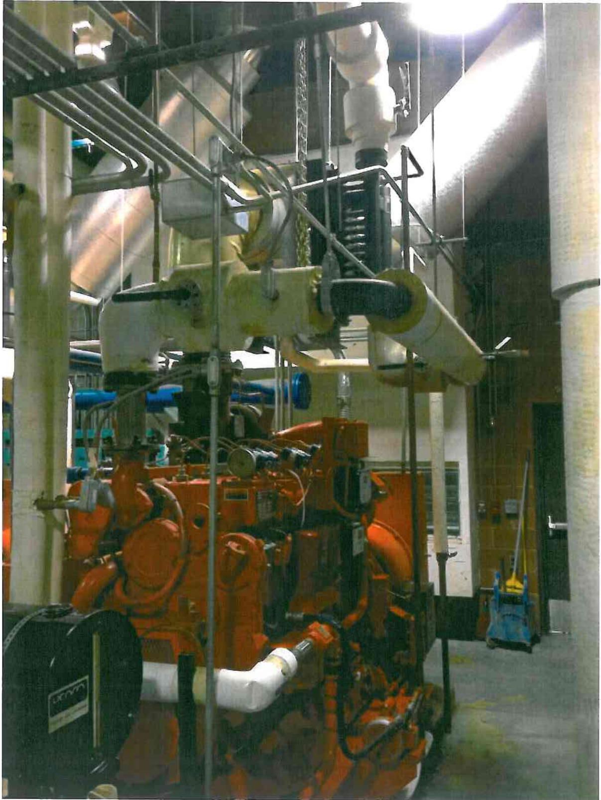
400 KW Engine Overall Views
