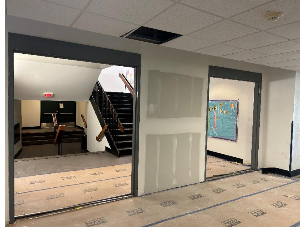
Egress Stair Doors
