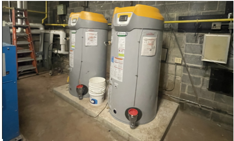
SDS - New Hot Water Tanks + New Concrete Pad
