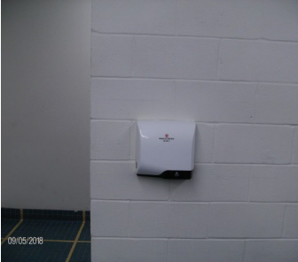
New Restroom Hand Dryers
