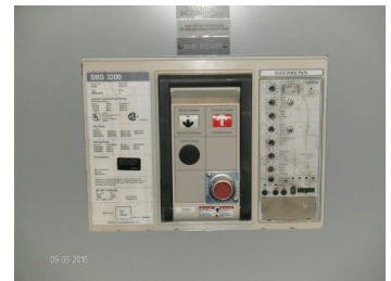
New Main Breaker Settings
