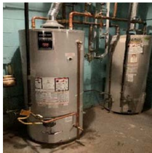
Domestic hot water heaters
