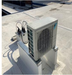
Ductless mini-split heat pump
