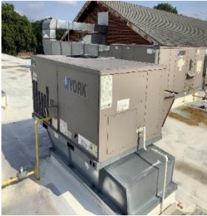
Packaged rooftop unit
