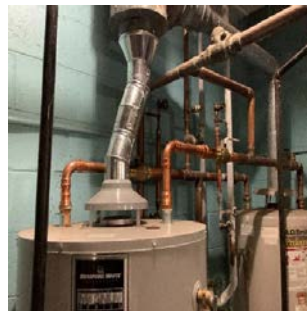
Domestic hot water piping without insulation
