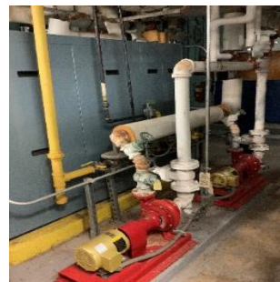
Hot water pumps
