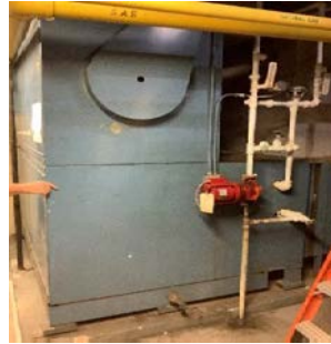
Air handling unit for cafeteria
