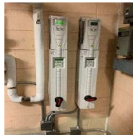
Variable frequency drive (VFD) controls
