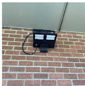
Wall-mounted LED fixture
