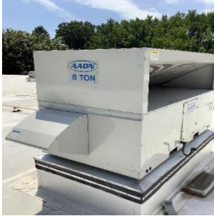
Packaged rooftop unit
