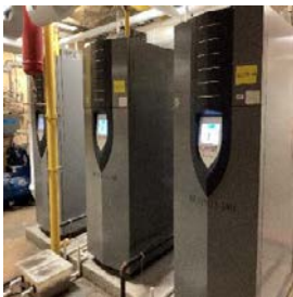
Three condensing hot water boilers
