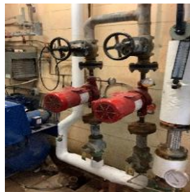
Hot water pumps
