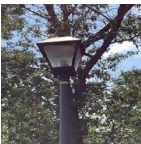
Pole-mounted fixture with LED lamp
