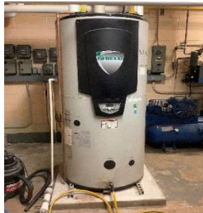
Condensing domestic hot water heater
