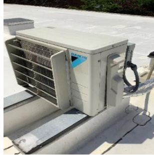
Ductless mini-split heat pump
