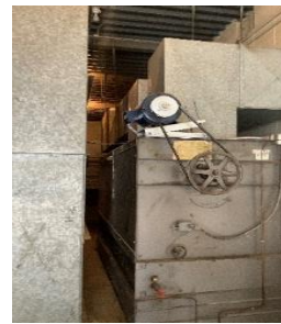
Air Handling Unit
