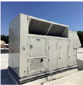
Packaged Rooftop Unit
