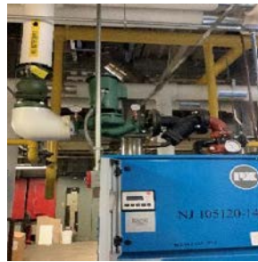
0.75 hp hot water pump
