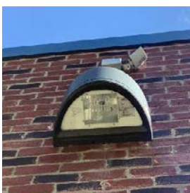
Wall-mounted fixture with metal halide lamps
