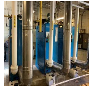
All three condensing hot water boilers
