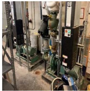
10 hp hot water pumps with VFD controls
