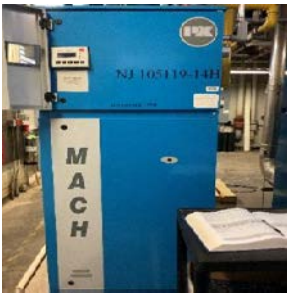
Condensing hot water boiler
