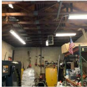
4' fixtures with fluorescent lamps
