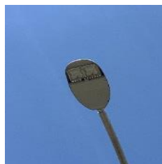
Pole mount fixtures
