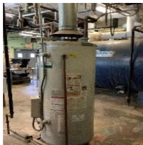
Hot water heater
