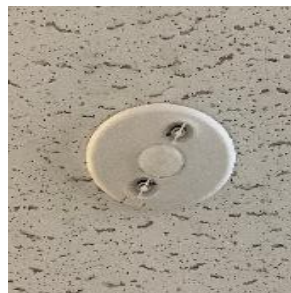
Remote occupancy sensor
