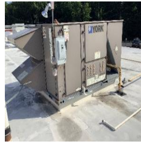
Gas-fired packaged rooftop unit
