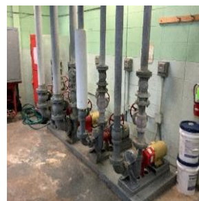
Hot water pumps
