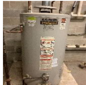
Gas storage water heater
