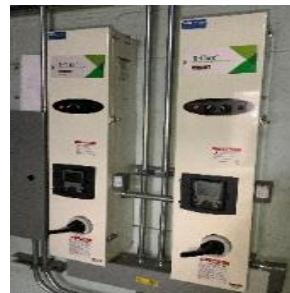
Hot water pump VFDs
