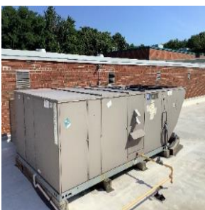
Rooftop packaged AC unit
