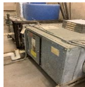
Indoor air-handling unit
