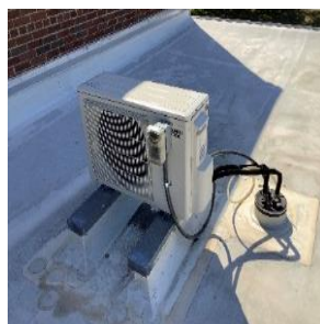
Ductless mini-split HP unit
