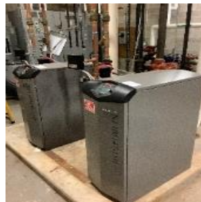
Condensing hot water boilers
