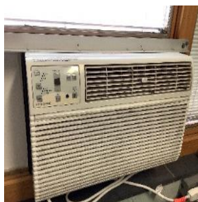
Window AC unit
