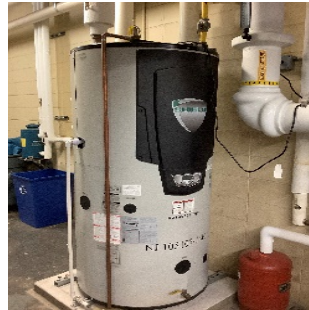
Hot water heater
