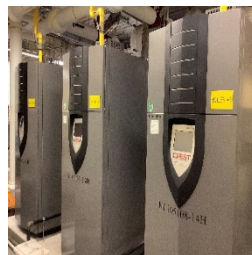
Hot water boilers
