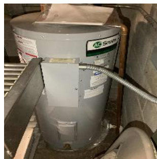
Electric domestic hot water heater
