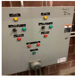
Sewage pump controls
