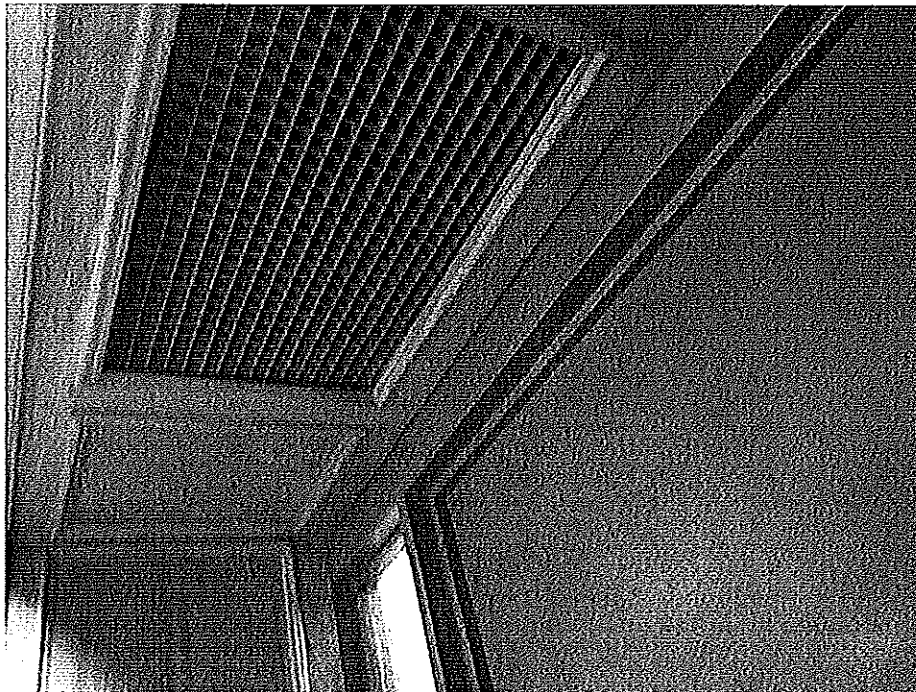
Return vent inside superintendent's suite
