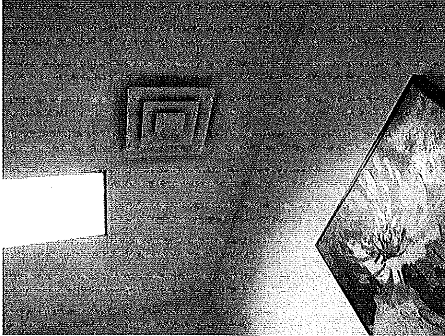
Supply vent from rooftop AHU
