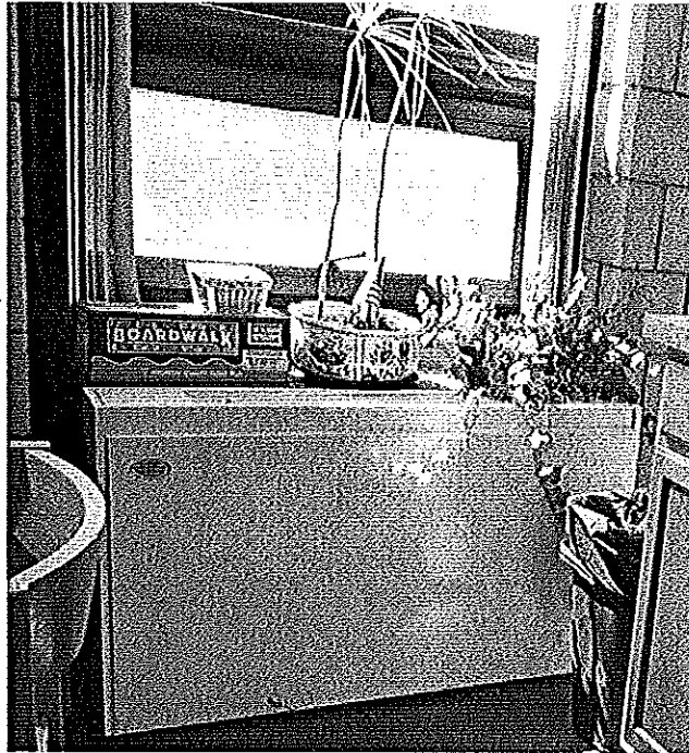
Univent blocked with items and plants
