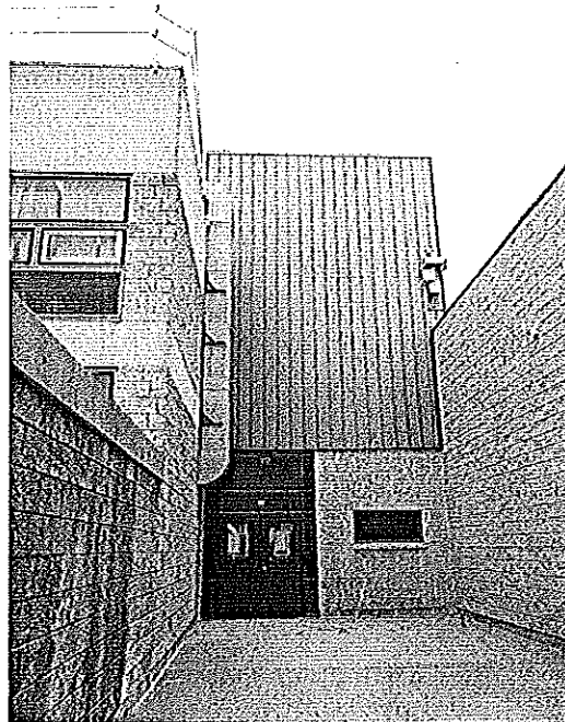
Signs of water staining on exterior walls
