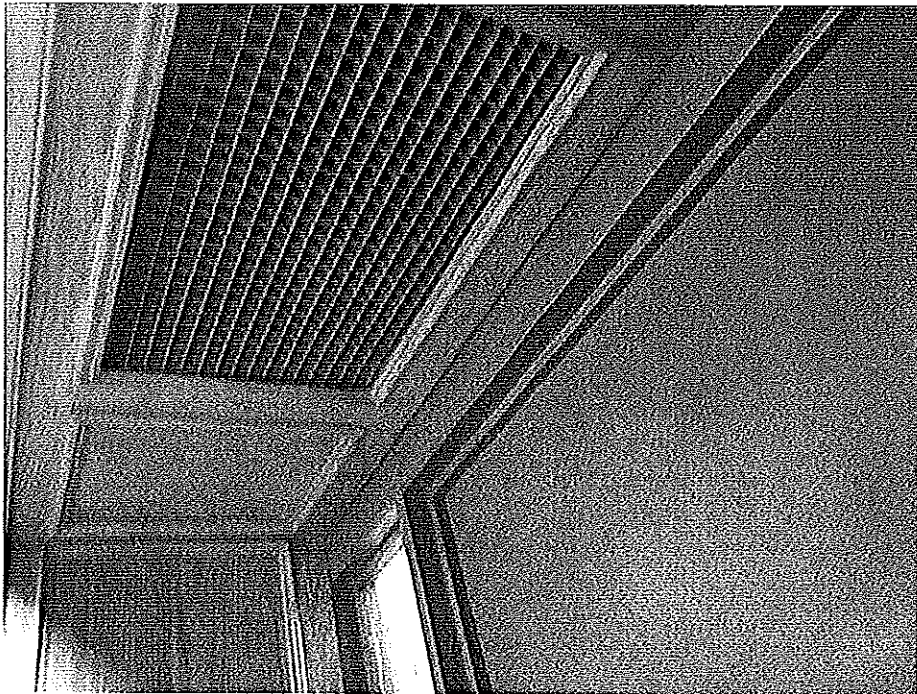
Return vent inside superintendent's suite
