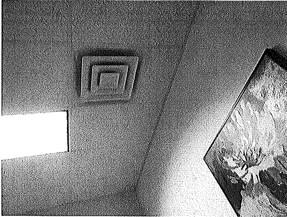
Supply vent from rooftop AHU
