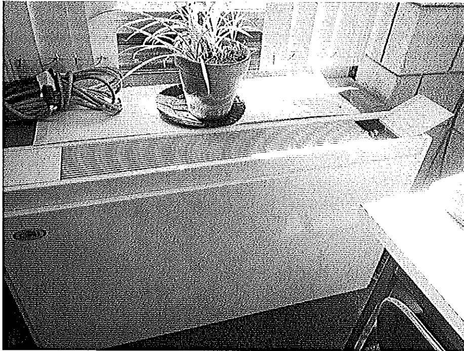
Typical univent, note plant on top
