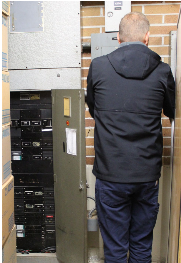
Replace outdated electrical panels (panel in photo is 65 years old)
