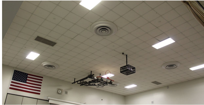
Energy-efficient light fixtures
