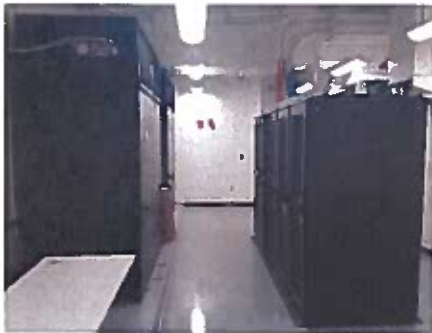
District Data Center
