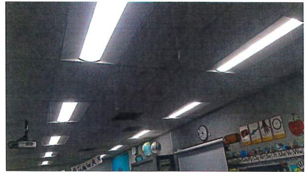
Typical LED lighting Upgrades throughout the District including interior and exterior lighting
