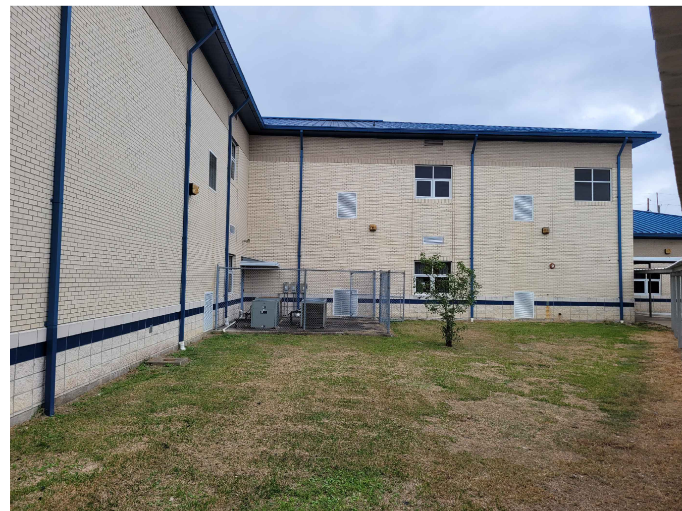
EXISTING EXTERIOR WALL PACKS
