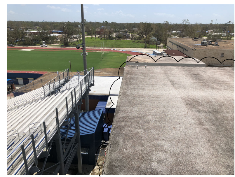
EXTERIOR PHOTO 553: DAMAGE TO EXISTING LOW SLOPE ROOF
