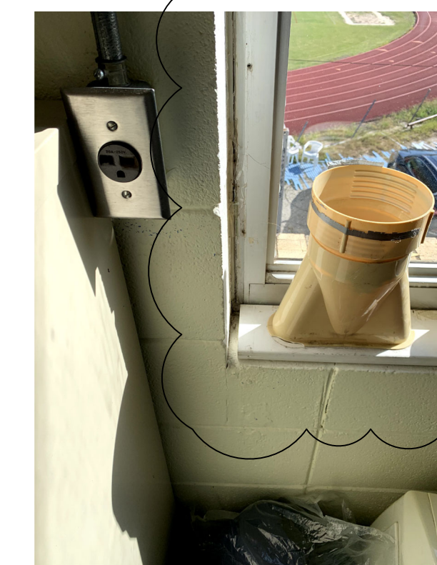
INTERIOR PHOTO: 537 DAMAGE TO EXISTING SEALANT AT WINDOW
