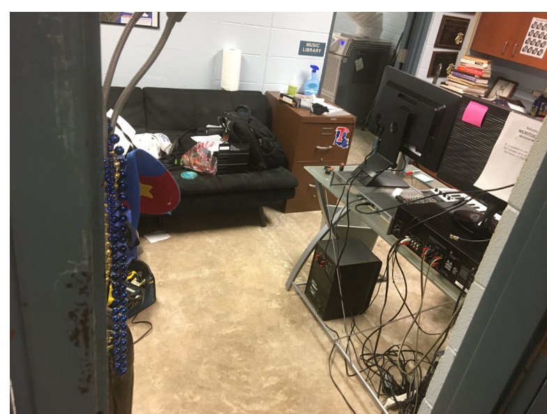
INTERIOR PHOTO: 515 DAMAGE TO EXISTING CARPET
