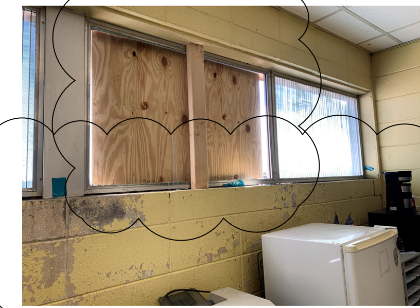
INTERIOR PHOTO: 529 DAMAGE TO EXISTING CMU, PAINTED FINISH AND WINDOW SEALANT
