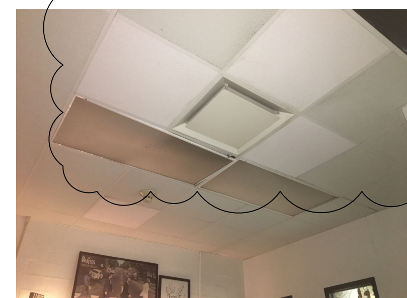
INTERIOR PHOTO: 505 DAMAGE TO EXISTING ACOUSTIC CEILING TILE
