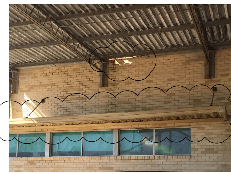
EXTERIOR PHOTO 556: DAMAGE TO EXISTING MTL ROOF & CANOPY
