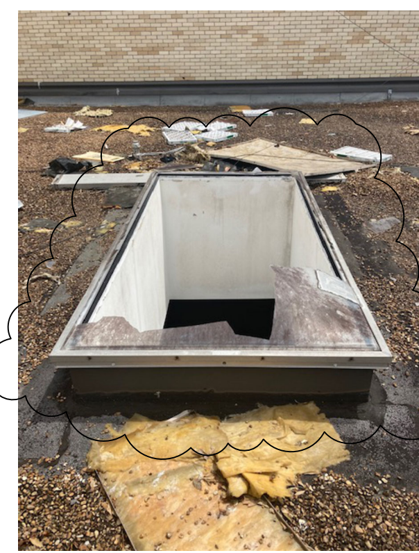
EXTERIOR PHOTO 552: DAMAGE TO EXISTING SKYLIGHT
