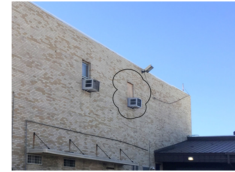
EXTERIOR PHOTO 562: DAMAGE TO EXISTING ALUM WINDOW
