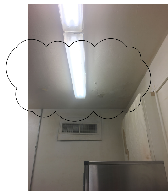
INTERIOR PHOTO: 502 DAMAGE TO EXISTING GYPSUM BOARD CEILING
