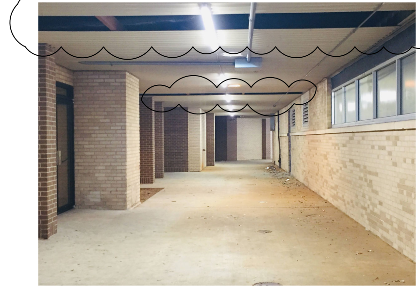
EXTERIOR PHOTO 560: DAMAGE TO EXISTING PREFIN MTL SOFFIT PANELS
