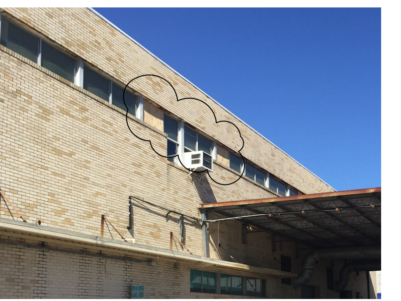
EXTERIOR PHOTO 558: DAMAGE TO EXISTING ALUM WINDOWS
