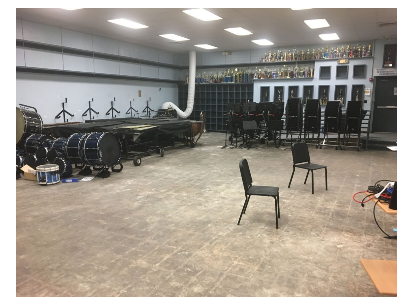
INTERIOR PHOTO: 511 DAMAGE TO EXISTING CARPET
