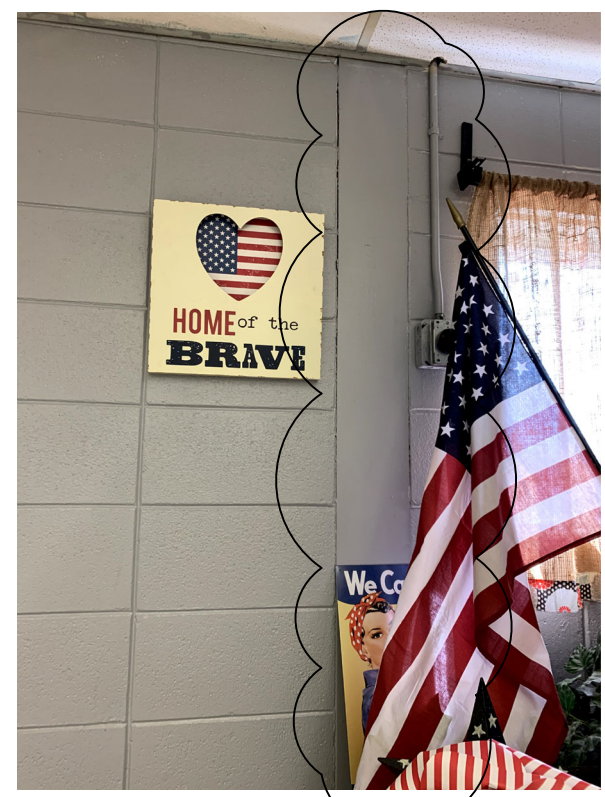
INTERIOR PHOTO: 524 DAMAGE TO EXISTING CMU WALL
