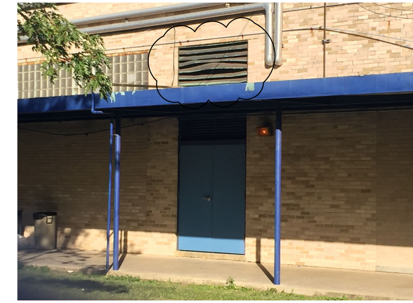
EXTERIOR PHOTO 561: DAMAGE TO EXISTING PREFIN MTL LOUVER
