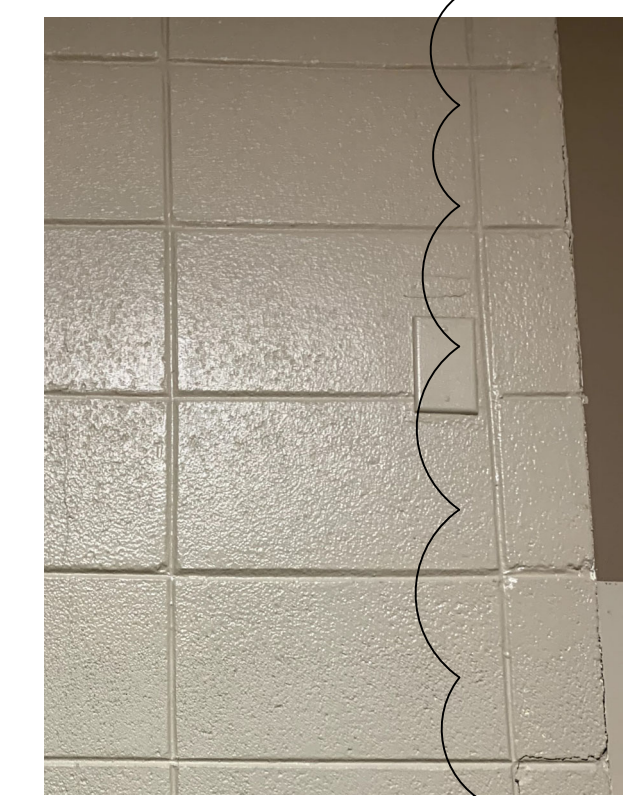
INTERIOR PHOTO: 519 DAMAGE TO EXISTING CMU WALL
