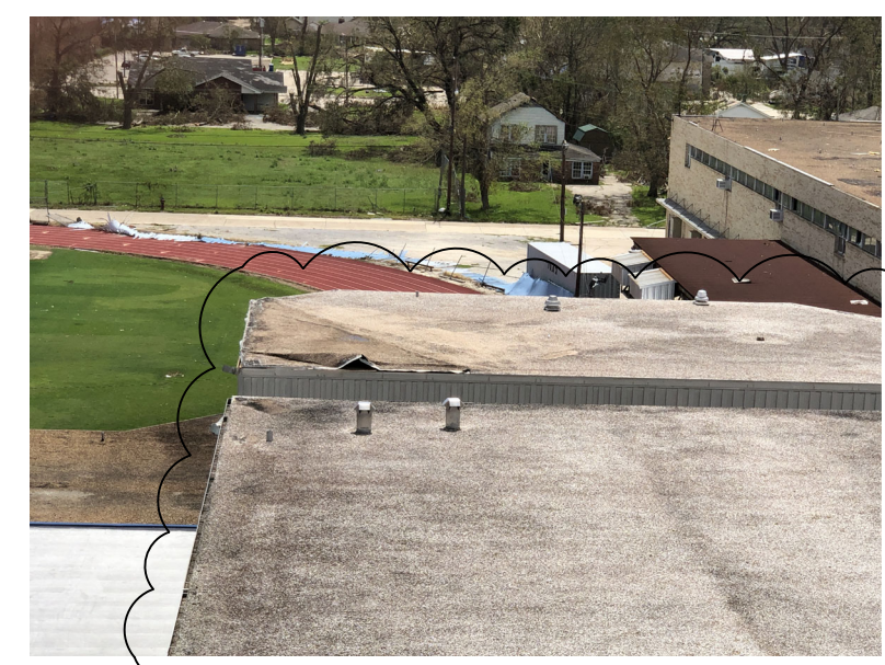
EXTERIOR PHOTO 554: DAMAGE TO EXISTING LOW SLOPE ROOF & EDGE TRIM
