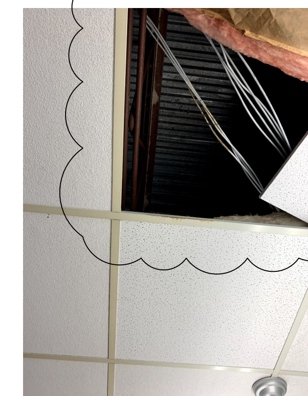
INTERIOR PHOTO: 536 DAMAGE TO EXISTING ACOUSTIC CEILING TILE
