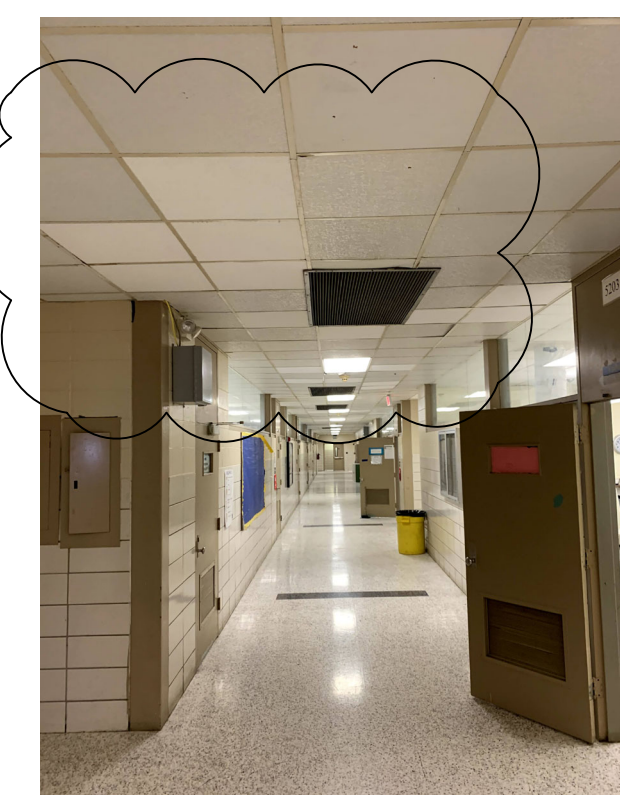
INTERIOR PHOTO: 520 DAMAGE TO EXISTING ACOUSTIC CEILING TILE
