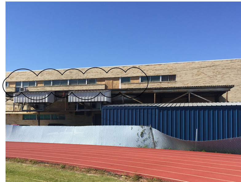
EXTERIOR PHOTO 559: DAMAGE TO EXISTING ALUM WINDOWS
