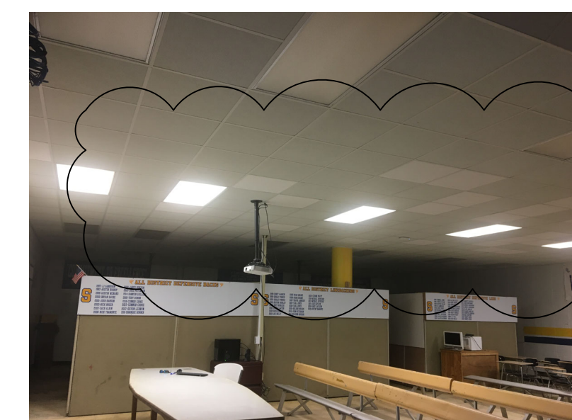
INTERIOR PHOTO: 517 DAMAGE TO EXISTING ACOUSTIC CEILING TILE
