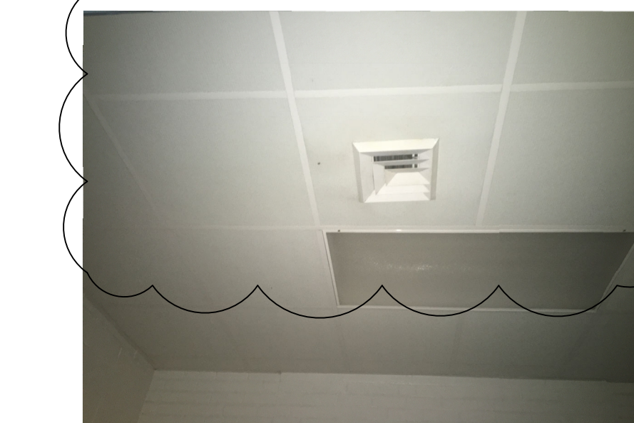
INTERIOR PHOTO: 509 DAMAGE TO EXISTING ACOUSTIC CEILING TILE
