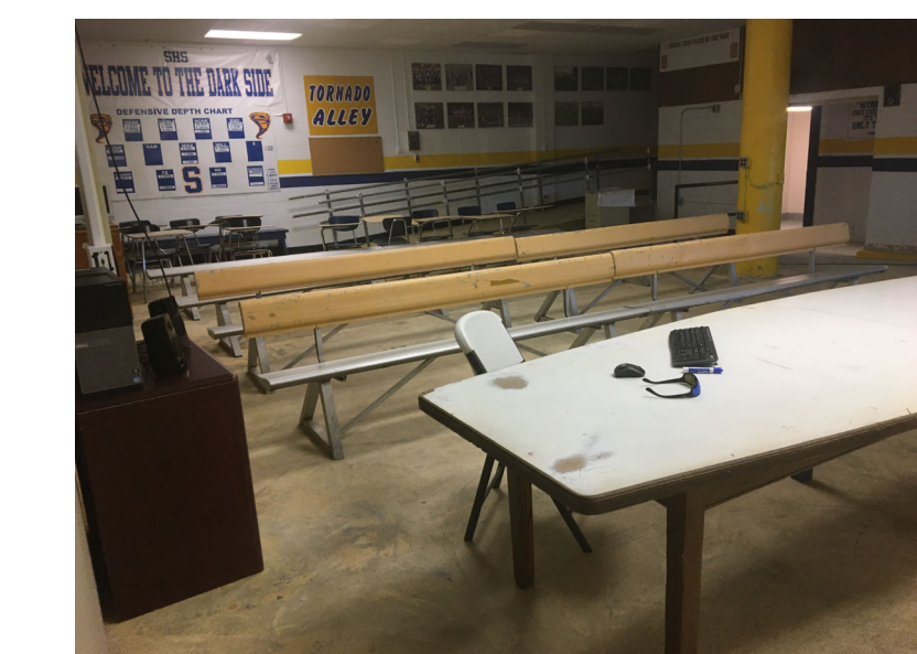
INTERIOR PHOTO: 516 DAMAGE TO EXISTING CARPET
