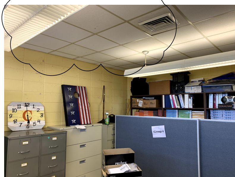
INTERIOR PHOTO: 531 DAMAGE TO EXISTING ACOUSTIC CEILING TILE
