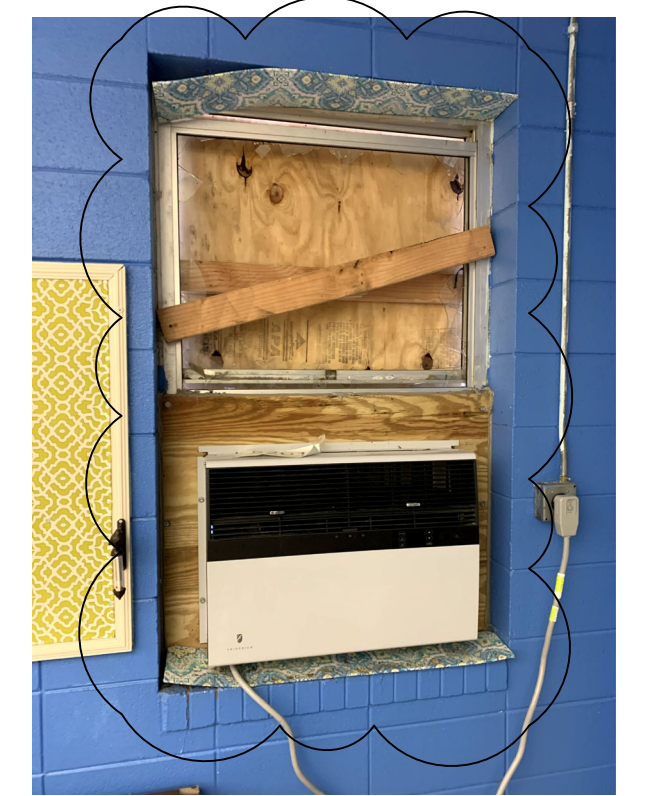
INTERIOR PHOTO: 522 DAMAGE TO EXISTING SEALANT AT WINDOW
