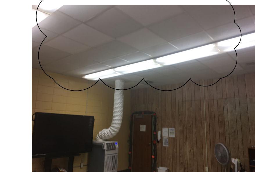
INTERIOR PHOTO: 510 DAMAGE TO EXISTING ACOUSTIC CEILING TILE
