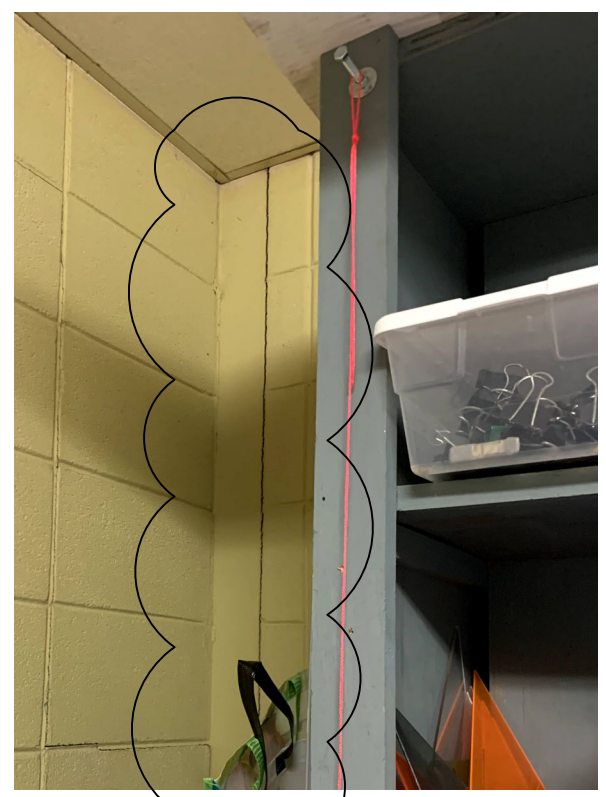
INTERIOR PHOTO: 523 DAMAGE TO EXISTING CMU WALL
