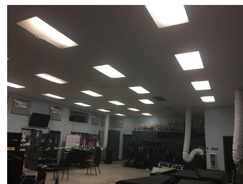
INTERIOR PHOTO: 513 DAMAGE TO EXISTING ACOUSTIC CEILING TILE
