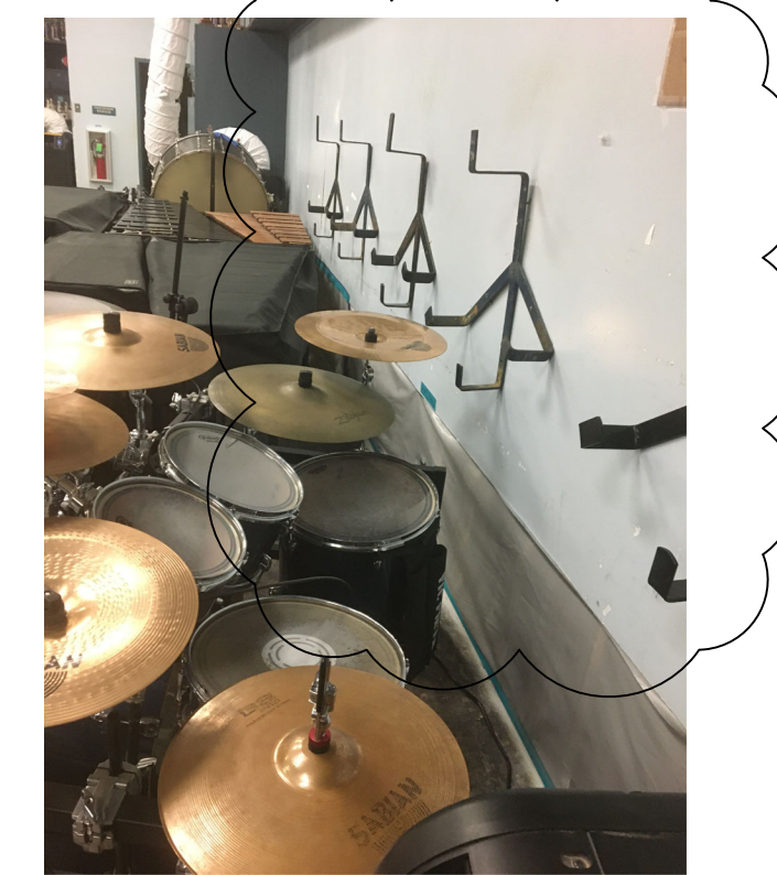
INTERIOR PHOTO: 512 DAMAGE TO EXISTING GYPSUM BOARD WALL & RESILIENT BASE
