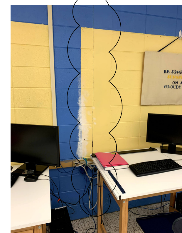
INTERIOR PHOTO: 521 DAMAGE TO EXISTING CMU WALL
