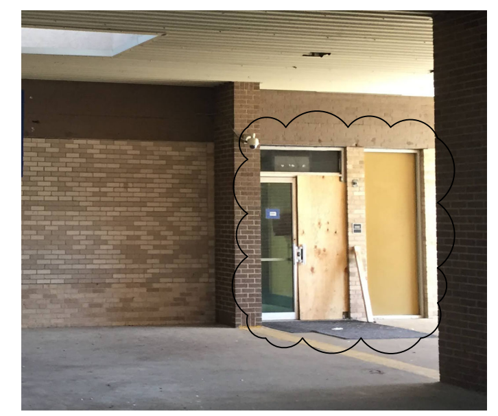
EXTERIOR PHOTO 557: DAMAGE TO EXISTING ALUM ENTRY DOOR AND METAL SOFFIT
