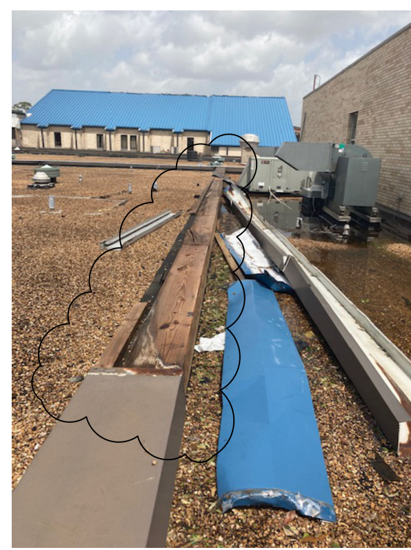
EXTERIOR PHOTO 551: DAMAGE TO EXISTING EXPANSION JOINT
