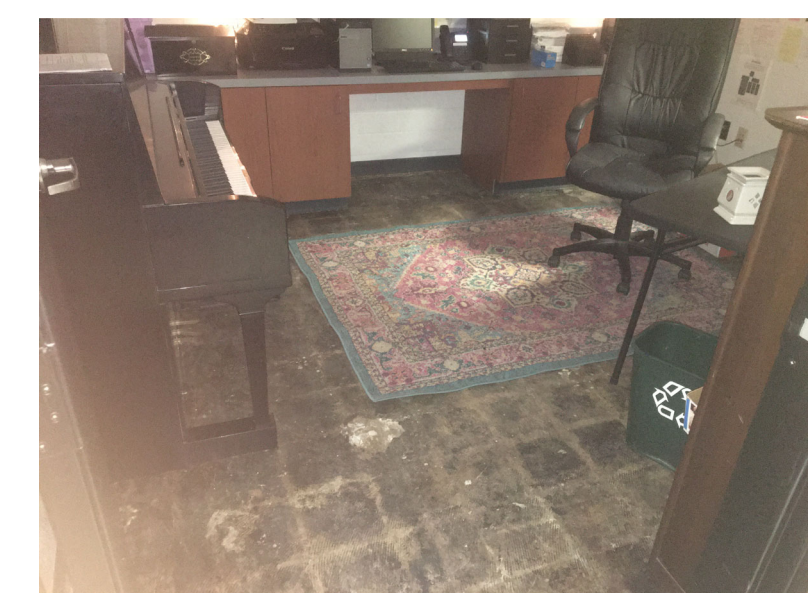
INTERIOR PHOTO: 504 DAMAGE TO EXISTING CARPET
