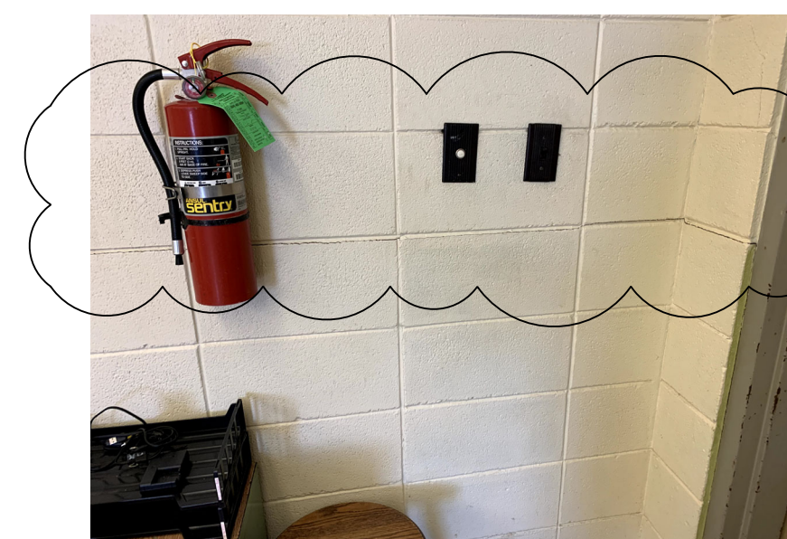
INTERIOR PHOTO: 534 DAMAGE TO EXISTING CMU WALL
