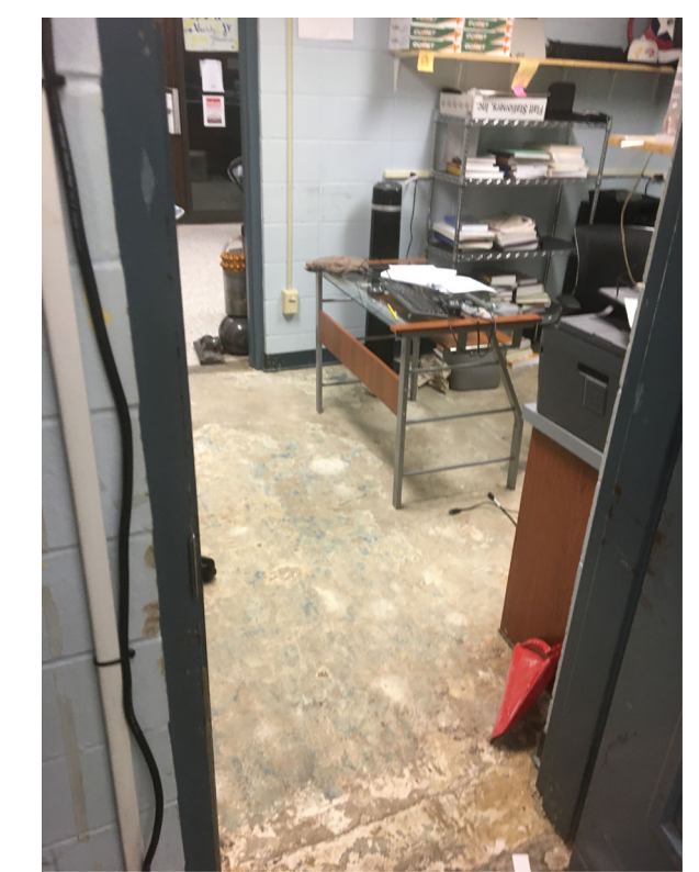
INTERIOR PHOTO: 514 DAMAGE TO EXISTING CARPET
