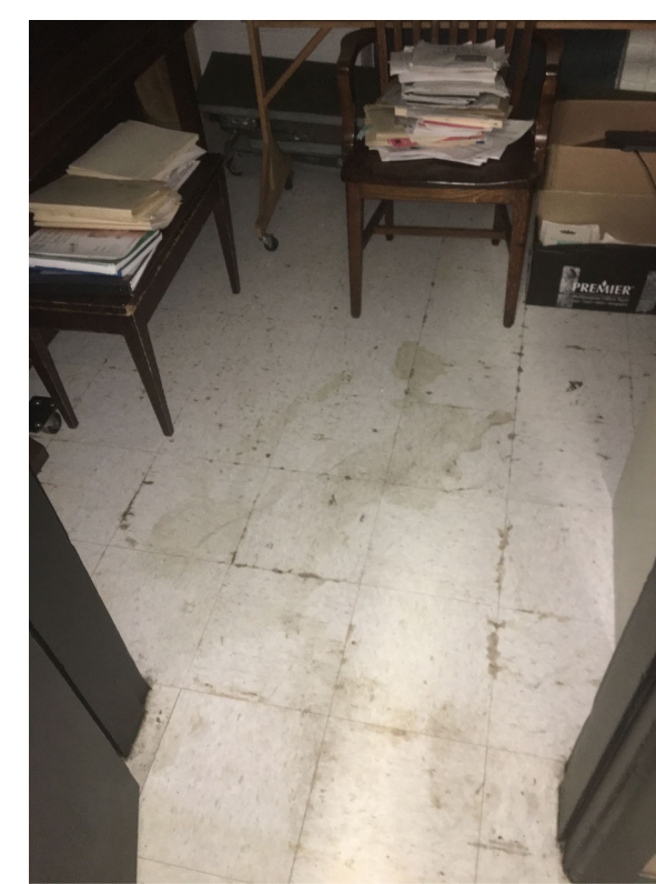
INTERIOR PHOTO: 506 DAMAGE TO EXISTING VCT FLOORING
