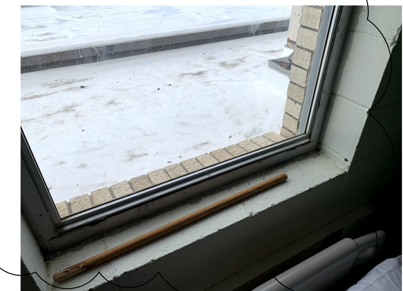
INTERIOR PHOTO: 539 DAMAGE TO EXISTING SEALANT AT WINDOW
