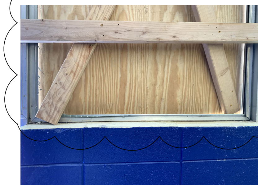
INTERIOR PHOTO: 535 DAMAGE TO EXISTING SEALANT AT ALUM WINDOW
