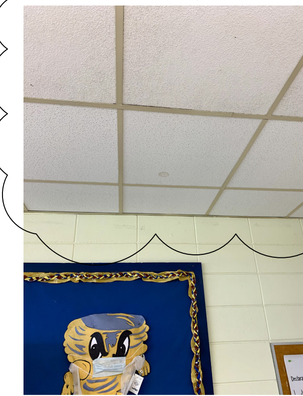
INTERIOR PHOTO: 538 DAMAGE TO EXISTING ACOUSTIC CEILING TILE
