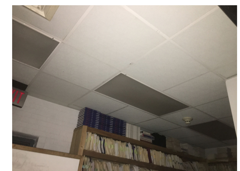
INTERIOR PHOTO: 507 DAMAGE TO EXISTING ACOUSTIC CEILING TILE
