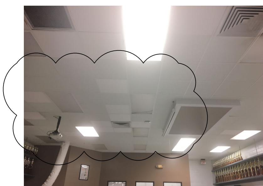
INTERIOR PHOTO: 503 DAMAGE TO EXISTING ACOUSTIC CEILING TILE
