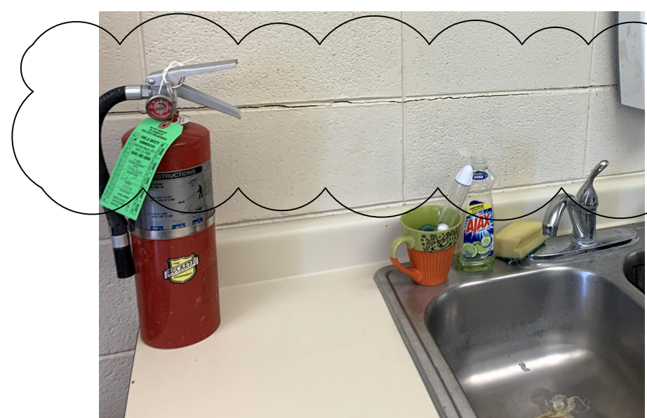
INTERIOR PHOTO: 532 DAMAGE TO EXISTING CMU WALL
