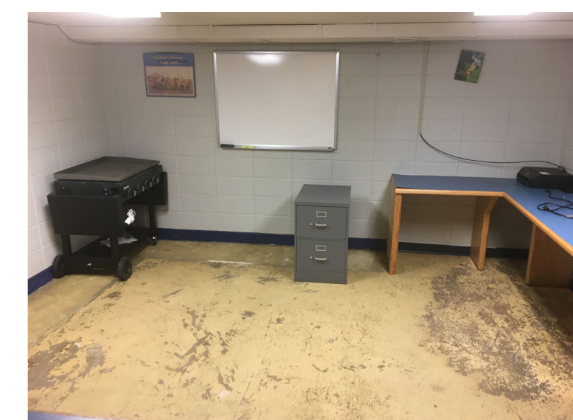
INTERIOR PHOTO: 518 DAMAGE TO EXISTING CARPET
