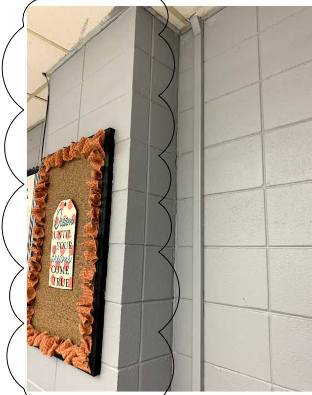
INTERIOR PHOTO: 525 DAMAGE TO EXISTING CMU WALL
