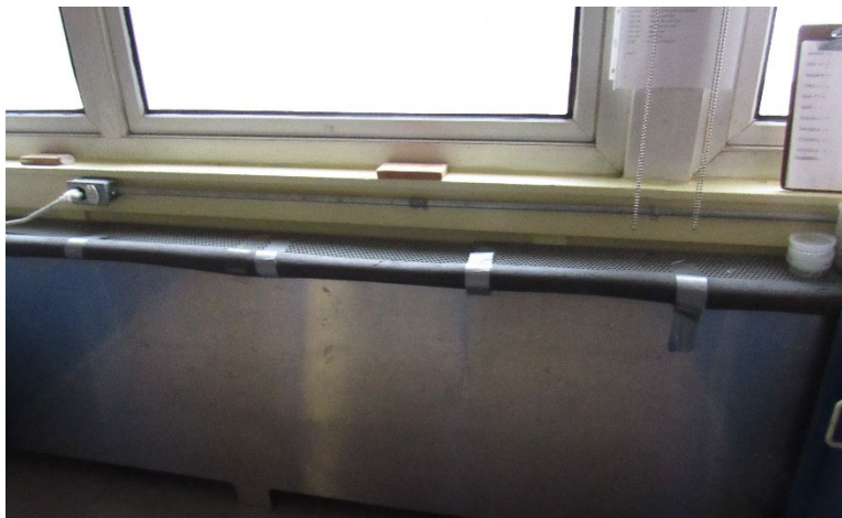
Archaic fin-tube heating element with foam duct-taped to it for protection.
