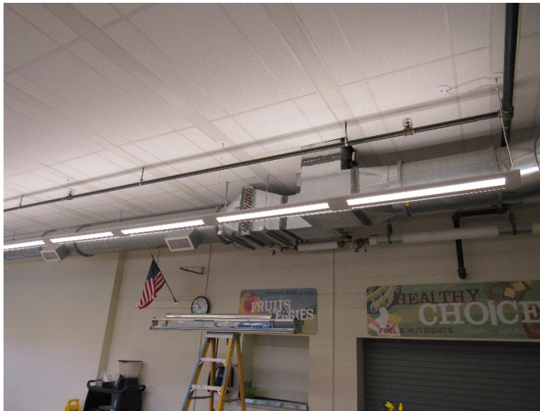
Mechanical system in the cafeteria.
