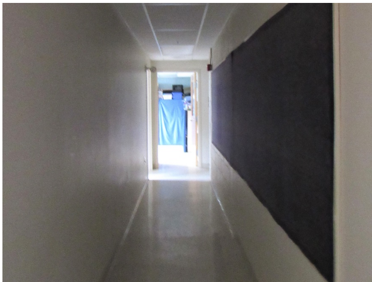
Basement corridor that is too narrow for code.
