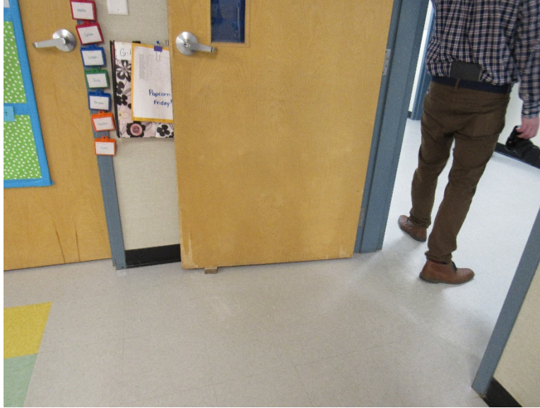
This school is mostly upgraded but some areas still show signs of wear such as this door that has been damaged by a door chock.
