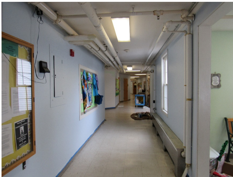
View of main lobby. Note the exposed heating pipes. The entrance to the main office is to the right.
