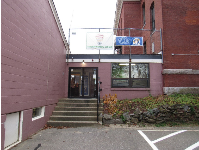
Front Entrance. Note the fencing on the roof to prevent unauthorized access.
