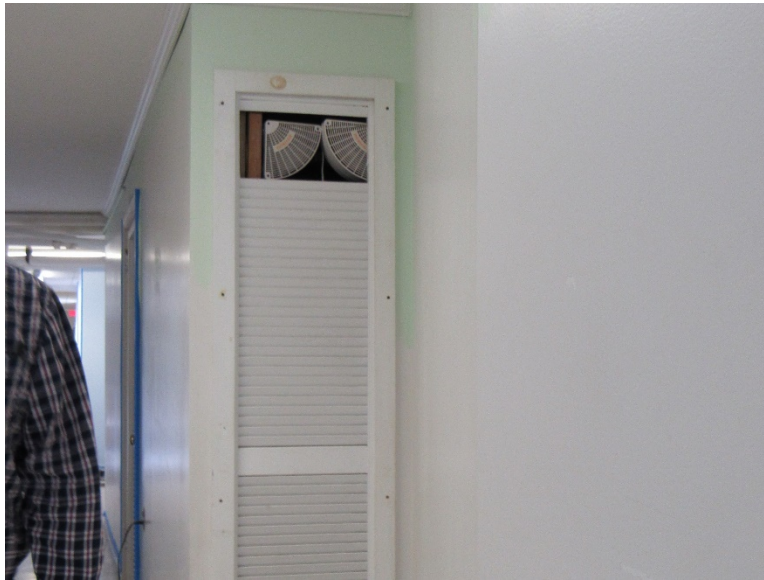
An unprotected vent into the corridor. Note the residential fans. Corridors need to resist the passage of smoke.
