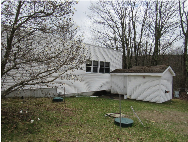
Exterior of kindergarten. Note the steep grades making a second exit difficult. Also, note the buried tanks.
