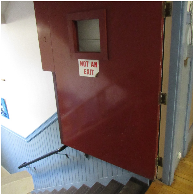
Doors at the top of the stair open over the stairs and have been notched to clear the stair lift making them not fire rated.
