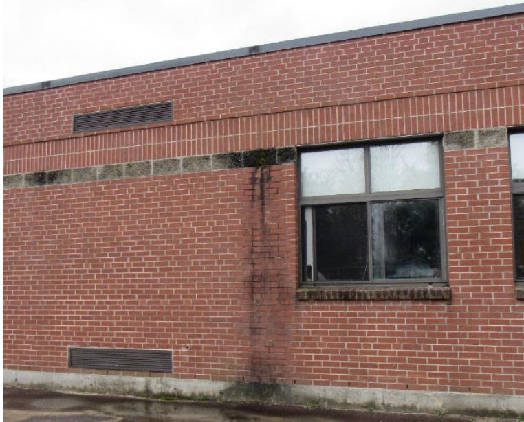
Exterior with mold from past moisture problems.
