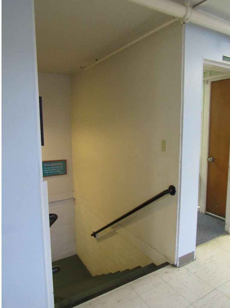
View of unprotected stair to basement.
