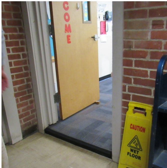
Entrance to a special needs classroom that is not handicap accessible.
