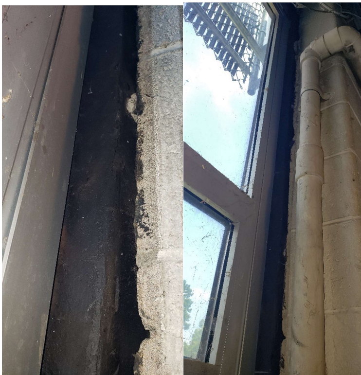
Asbestos-Containing Black Damp-proofing in Wall Cavity by Window/Louver Vent
