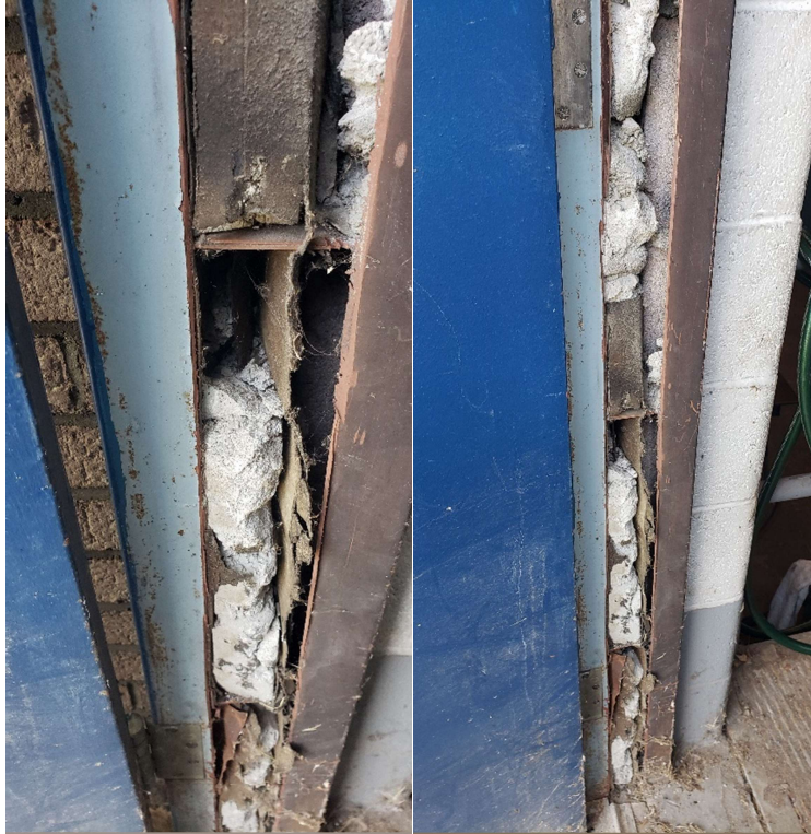
Asbestos-Containing Black Damp Proofing in Wall Cavity by Door 24
