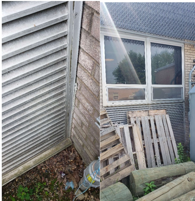
Window/Louver Vent with Asbestos Containing Caulking Compound
