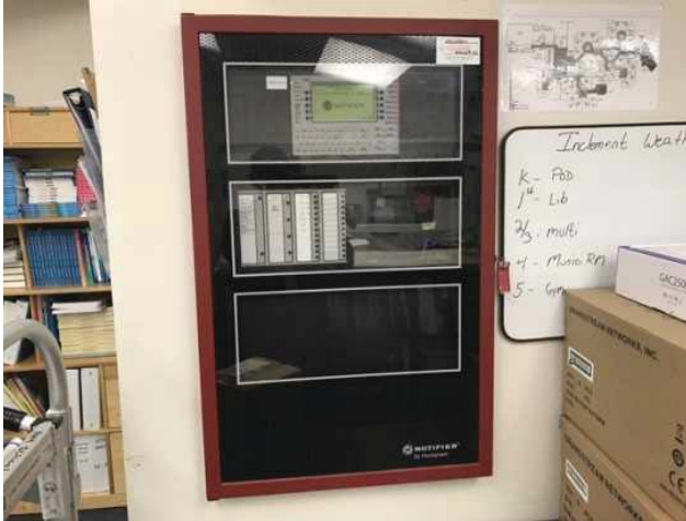
25 - FIRE ALARM PANEL
