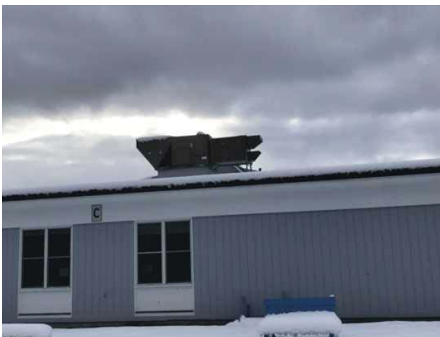
17 - ROOFTOP PACKAGED UNIT
