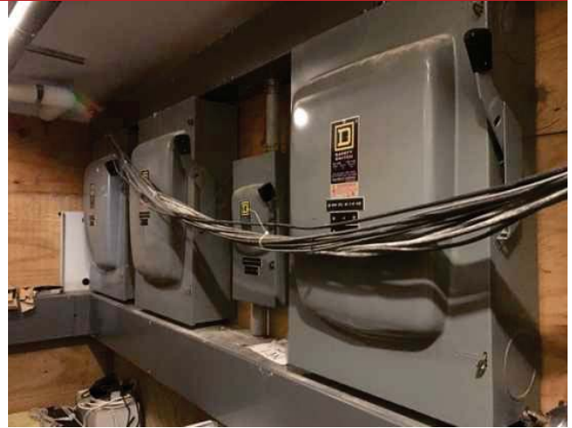
26 - MAIN DISCONNECT SWITCHES
