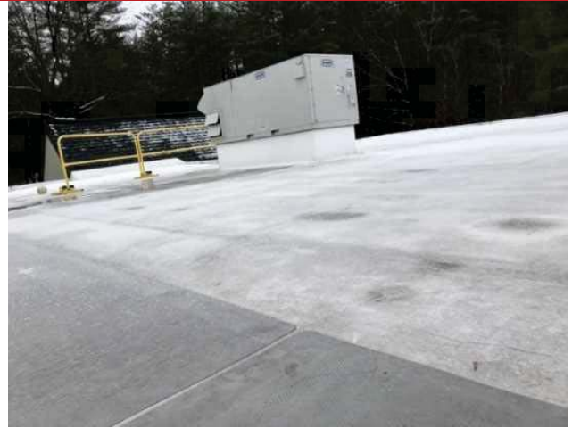
20 - ROOFTOP PACKAGED UNIT
