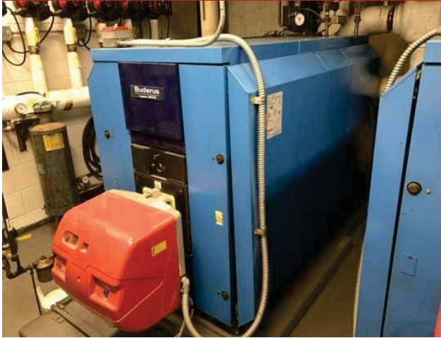
19 - HOT WATER BOILER
