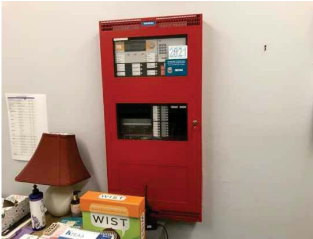
27 - FIRE ALARM PANEL
