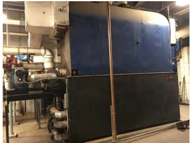
16 - WOOD FIRE PLANT
