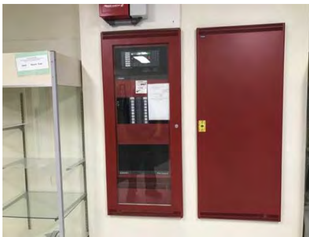
27 - FIRE ALARM PANEL
