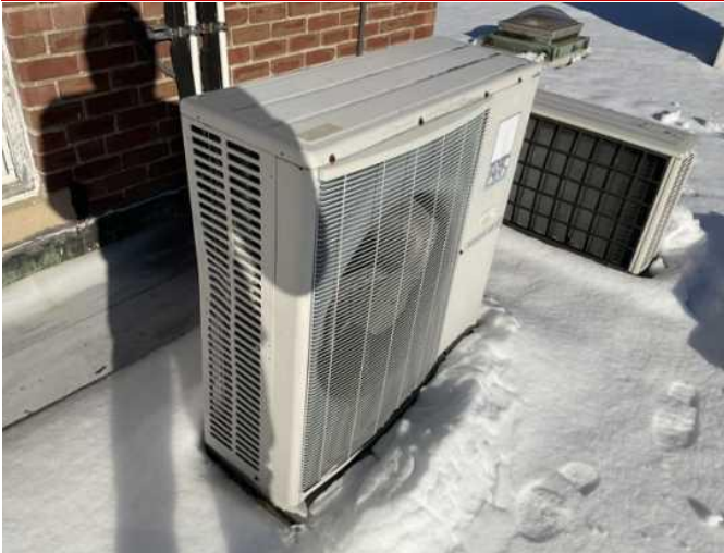
25 - DUCTLESS SPLIT SYSTEM
