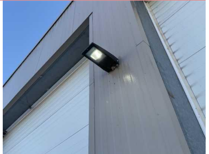
32 - EXTERIOR LIGHT FIXTURE
