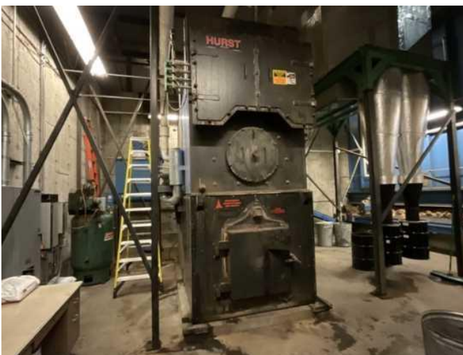
17 - WOOD CHIP BOILER
