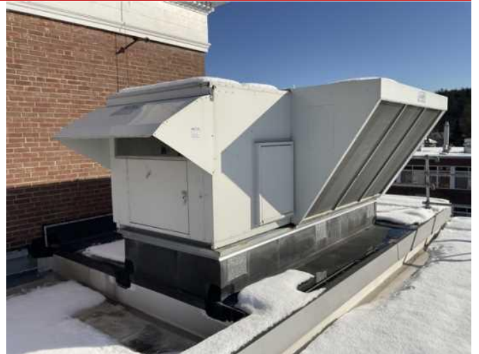
20 - ROOFTOP PACKAGED UNIT
