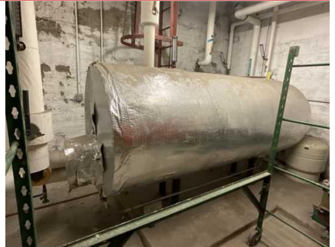
26 - DOMESTIC STORAGE TANK
