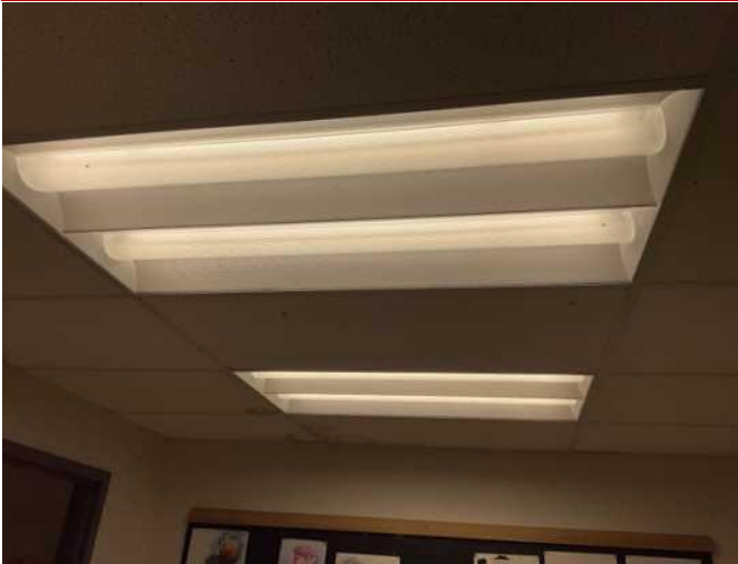
31 - INTERIOR LIGHTING SYSTEM
