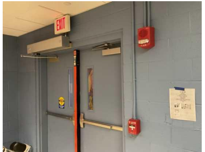
34 - FIRE ALARM SYSTEM
