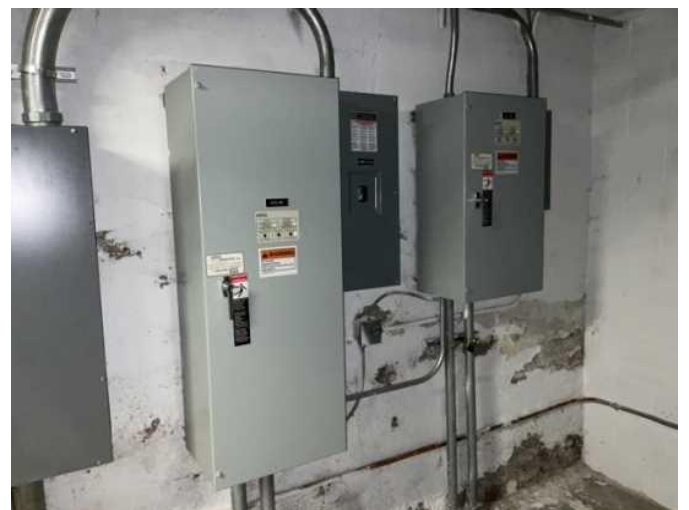
30 - AUTOMATIC TRANSFER SWITCHES
