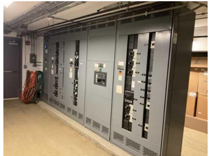
28 - MAIN ELECTRICAL EQUIPMENT
