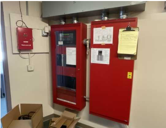
33 - FIRE ALARM PANEL
