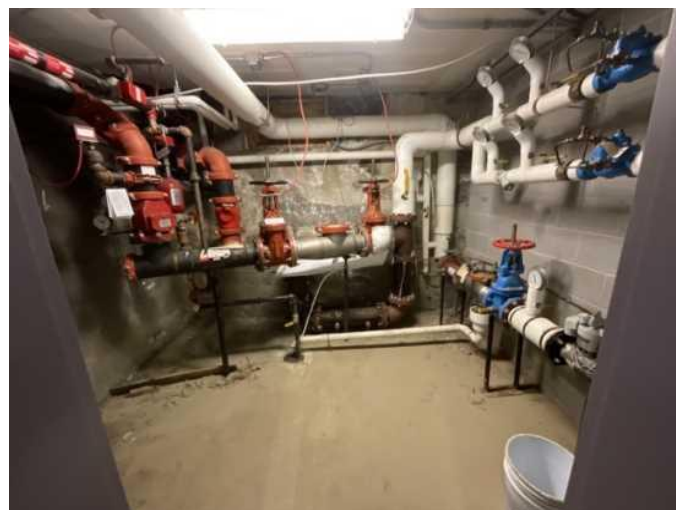
36 - FIRE SUPPRESSION SYSTEM
