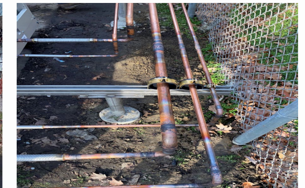
Chiller piping & fencing
