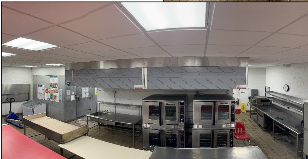
Pomona MS – Kitchen Hood & Equipment Photos
