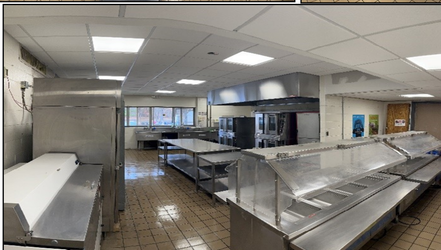
Margetts ES – Kitchen Hood & Equipment Photos
