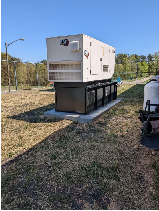
Generator – Widewater ES
