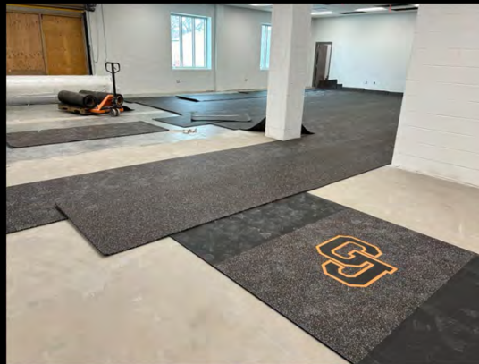
Weight Room Flooring
