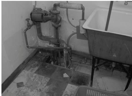
Piping leaks that are causing water damaged floors
