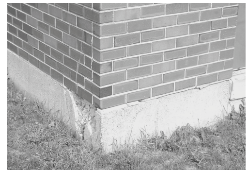
Cracked concrete foundation walls undermining masonry veneer
