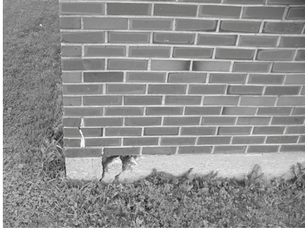
Cracked concrete foundation walls undermining masonry veneer
