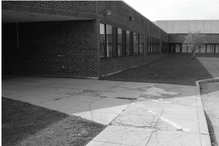
Damaged sidewalks, concrete, and curbs in need of replacement
