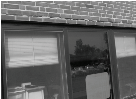
Masonry cracks with possible damaged lintels
