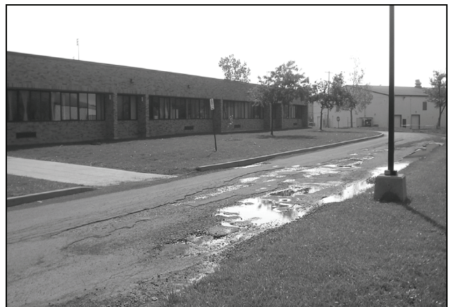
Above: Poor condition of paving at the High School loop road.
