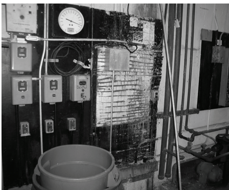
Water leaks, an indication of possible infrastructure damage and/or roof leaks
