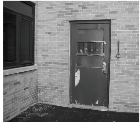
Damaged door in need of replacement
