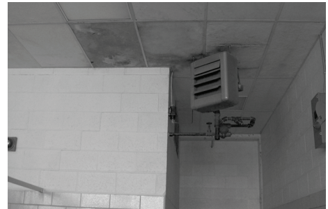
Water damage in girls locker room, which is an indicator of possible infrastructure damage and/or roof leaks
