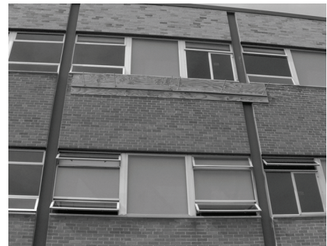
Temporary fix for damaged brick
