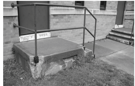
Badly damaged concrete in need of repair that is undermining the foundation of the landing
