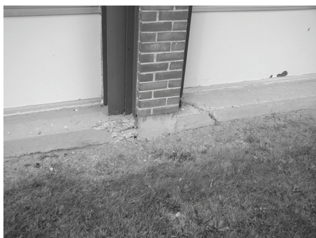
Cracks in foundation that will eventually undermine the column
