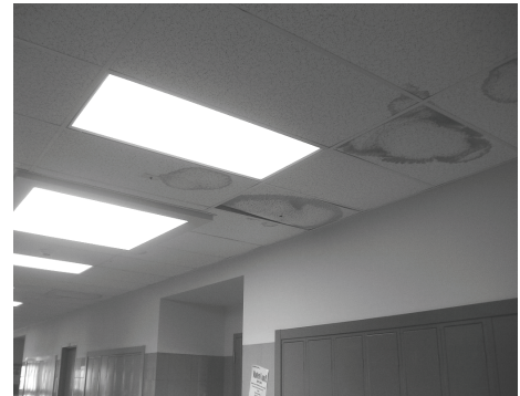
Water damaged ceiling tiles, an indication of possible infrastructure damage and/or roof leaks
