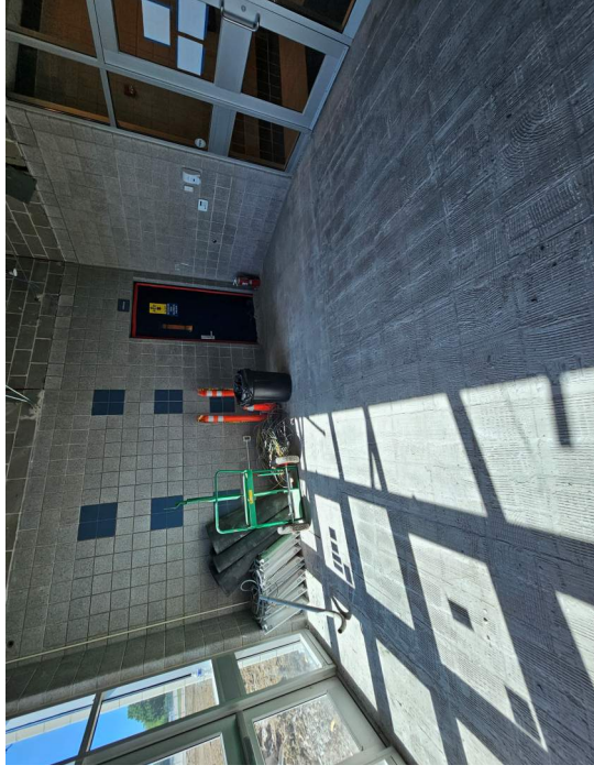
SVMS - Interior Demo
