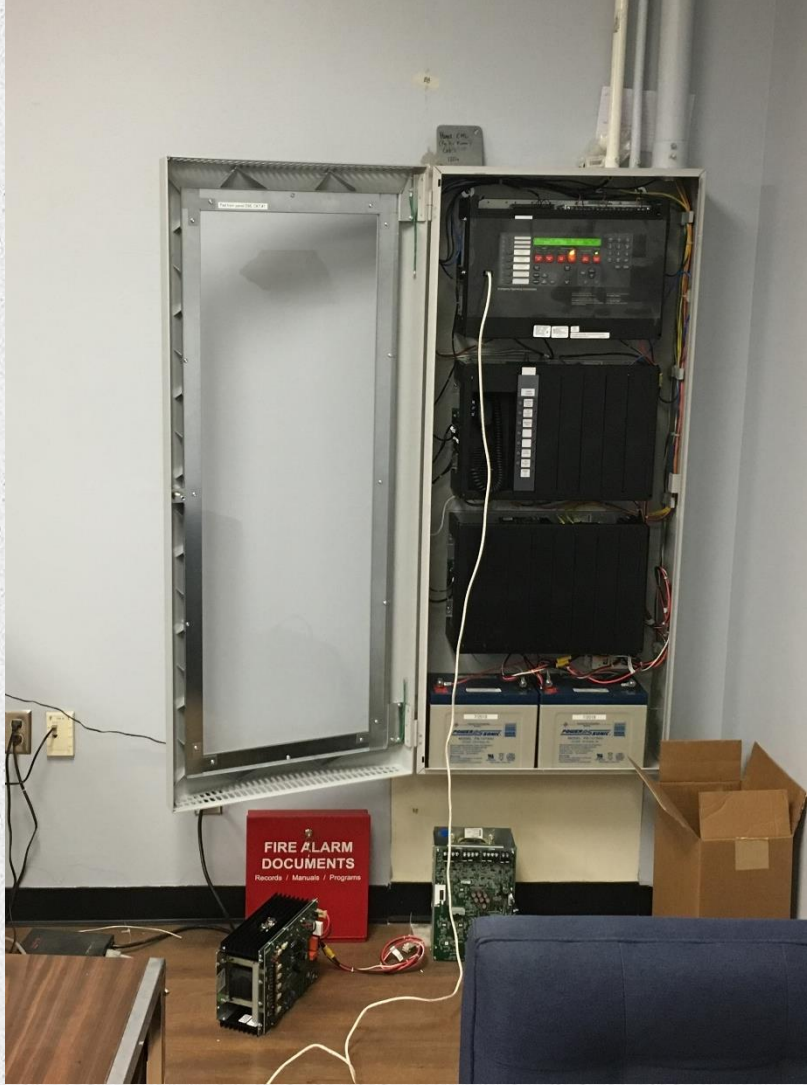
Fire Alarm System Replacement $400,000
