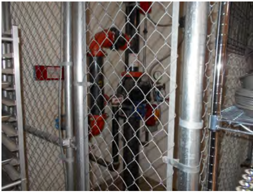
Canutillo_Central_Office Warehouse Sprinkler system
