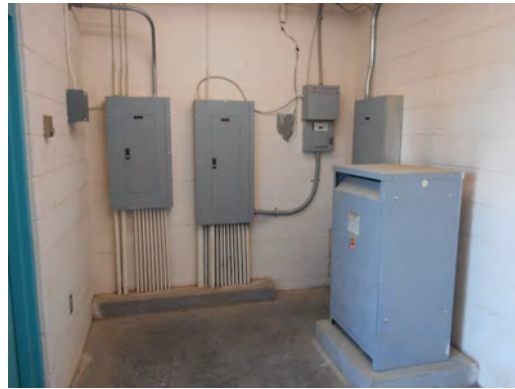
Childress ES_Electrical panels
