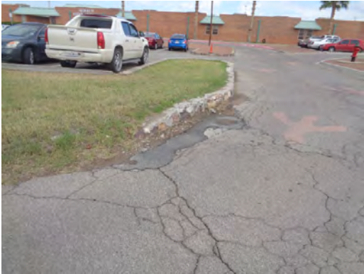
Alderete_MS Parking lot damaged, replace and restripe
