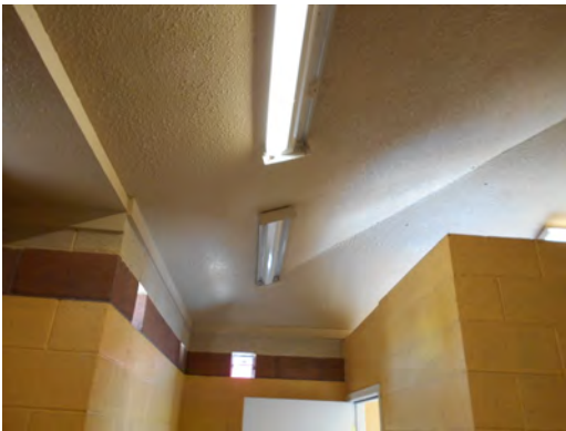
Canutillo ES_Light fixtures failing
