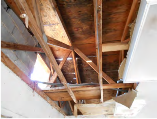
Lone_Star_Buildings Cottage 1, Interior damage
