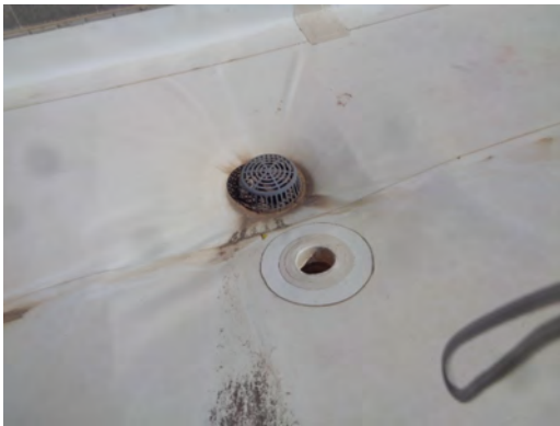
Canutillo ES_Roof debris covers, stainers are missing
