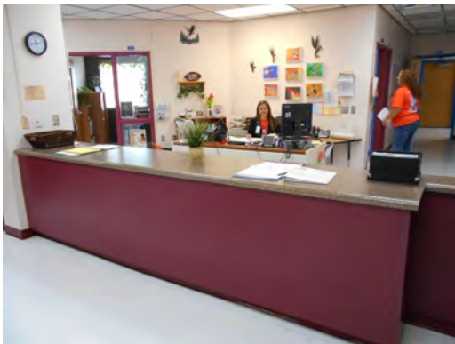
Davenport_ES Counter is not ADA Compliant
