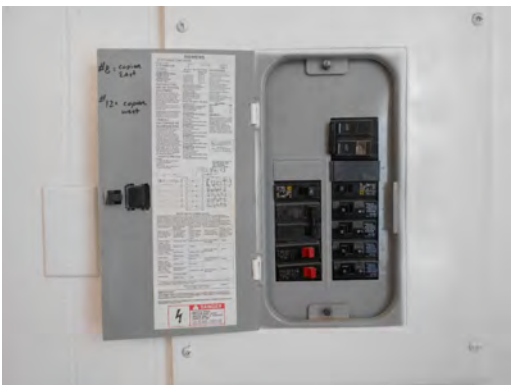
NW_Early_College_Campus Electrical panelboard in classrooms
