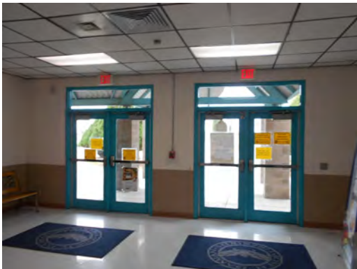
Damian_ES Entry doors require ADA assist device
