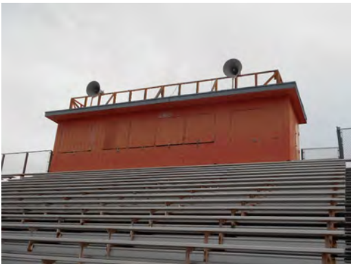
Canutillo_MS Press Box, abandoned, not structurally safe
