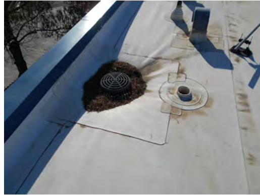
Davenport_ES Clean roof and install debris covers on overflow drains
