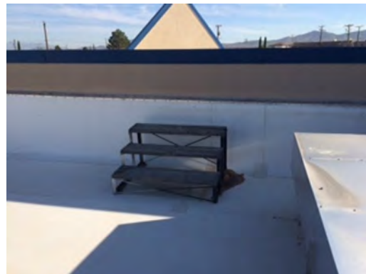
Davenport_ES unsafe roof access
