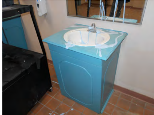
Lone_Star_Buildings Unused bld, interior vandalism damage
