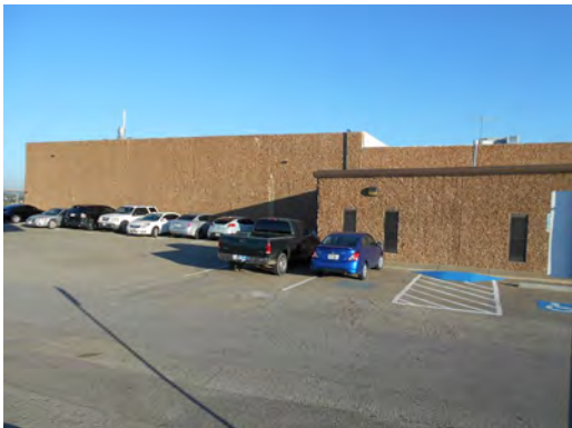
Canutillo_Central_Office No safe roof access from upper level (roof hatch) to to the lower level over offices
