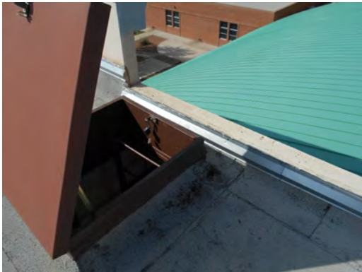
Alderete_MS Science building, roof hatch system opens onto a ledge. Safety fall hazard. Orient the hatch system correctly
