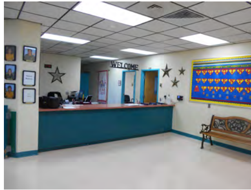
Childress ES_Main Office counter exceeds max ADA height
