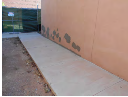
NW_Early_College_Campus Exterior paint deficiency
