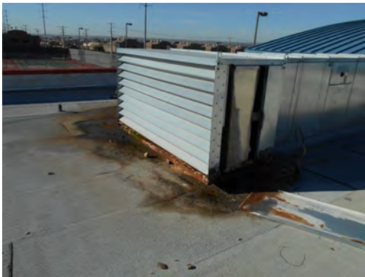
Canutillo_HS Ag 1 Building, evaporative cooler failure
