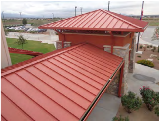
Garcia_ES Gutter joints leak, seal joints
