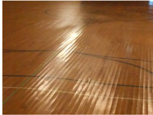
Canutillo_HS Gym floor water damage
