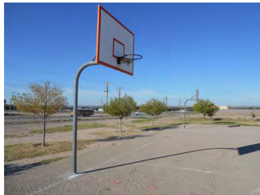
Childress ES_Basketball court asphalt paving requires replacement
