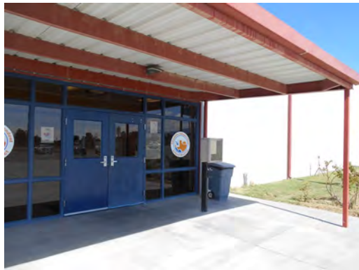
Canutillo_Facilities_Transportation Entry doors not ADA Compliant
