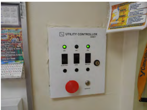
Canutillo_HS Gas control modules out of date and not functional for class use
