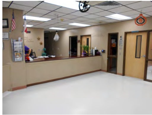
Damian_ES Admin countertop is not ADA compliant
