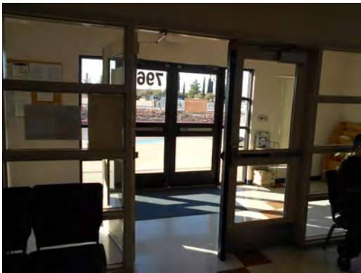
Canutillo_Central_Office Main Entry not ADA Compliant
