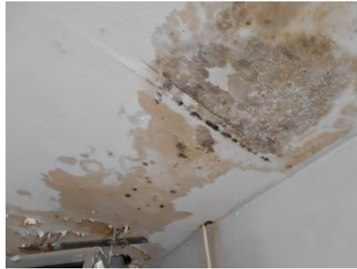
Lone_Star_Buildings Cottage 1, Interior Damage
