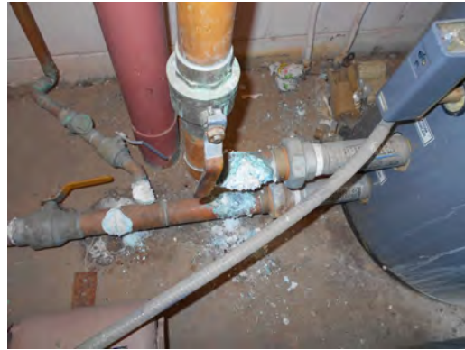
Damian_ES Mechanical room, needed water pipe repairs
