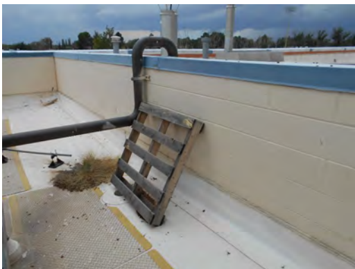
Canutillo_MS Unsafe roof access, wood pallet used as ladder
