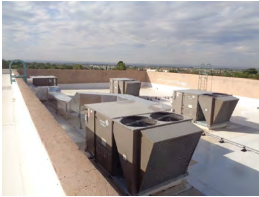
Alderete_MS Main building, seal parapet walls and recaulk flashing joints
