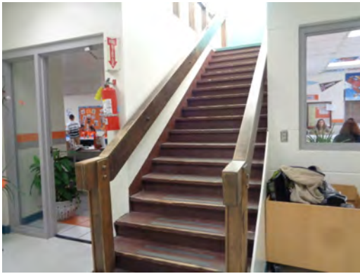
Alderete_MS Main building, handrails not ADA compliant
