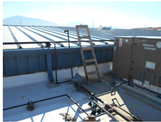
Canutilo ES_Unsafe roof access 2
