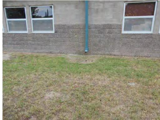
Damian_ES Splashpads required to prevent erosion
