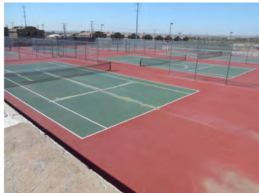
Canutillo_HS Basketball and tennis courts pavement failure
