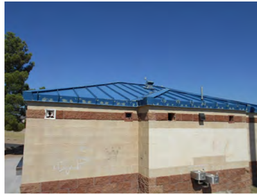
Canutillo ES_Metal roof should be replaced
