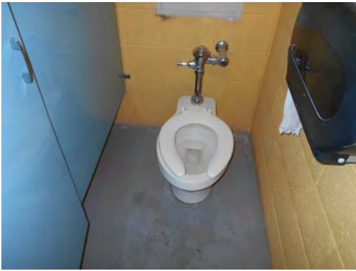
Canutillo ES_Interior CMU needs repainting
