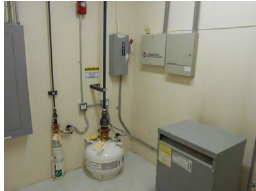
Canutillo_Central_Office Computer Room fire suppression
