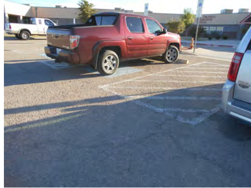
Childress ES_ADA accessible parking spaces not properly striped
