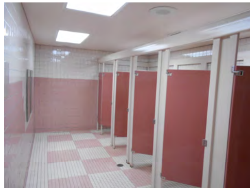
Childress ES_Restroom Toilet Partitions
