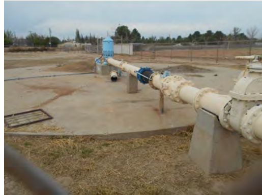
Canutillo_MS Lift Station
