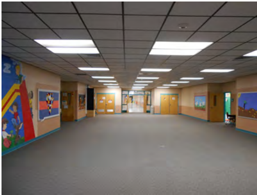
Childress ES_Carpet requires replacement
