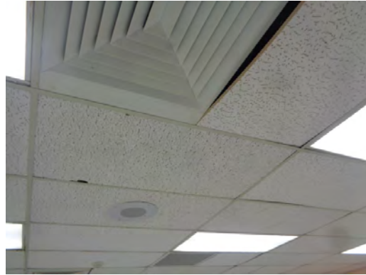
Alderete_MS Ceiling grid and time system
