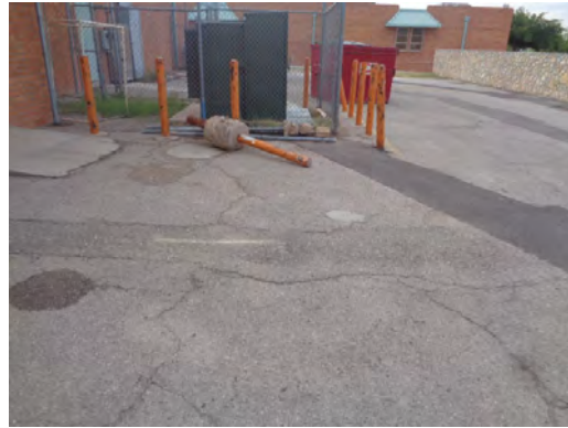
Alderete_MS Bollard damaged
