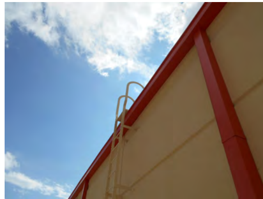
Alderete_MS New Gym building, the roof ladder needs additional safety rails. The ladder is at the edge of a steep exterior wall with no parapet or additional protection.
