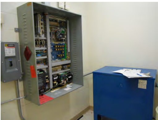
Canutillo_HS Elevator H Wing not working
