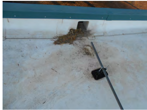
Childress ES_Roof requires cleaning
