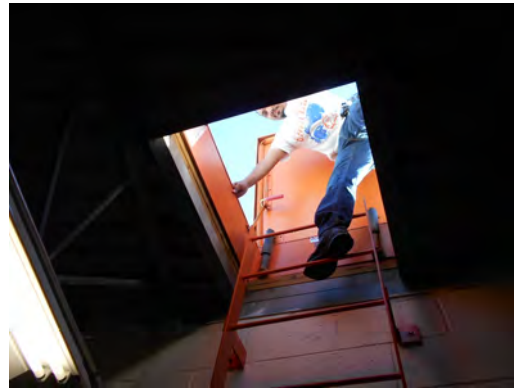
Canutillo_HS Roof ladder deficiencies
