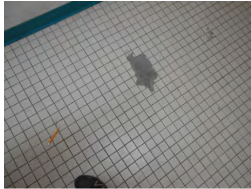
Childress ES_Damaged ceramic tile
