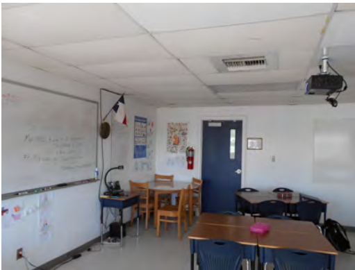
NW_Early_College_Campus Classrooms need to be painted
