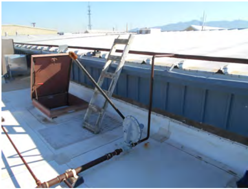
Canutilo ES_Unsafe roof access 1
