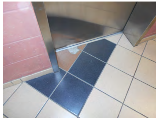
Canutillo_HS Ceramic floor tile deficiencies throughout building
