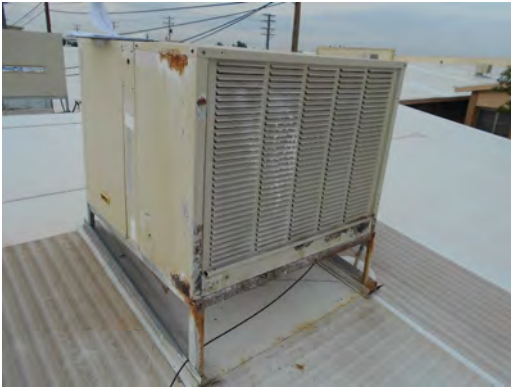
Lone_Star_Buildings Main Bld Evaporative coolers
