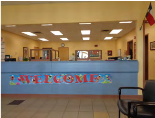
Canutillo ES_Countertop does not meet ADA
