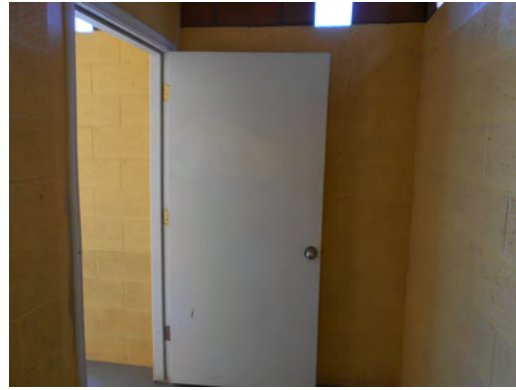
Canutillo ES_Interior doors need repainted
