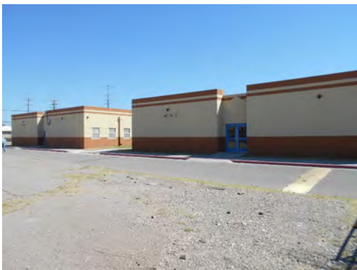
Canutillo ES_Site drainage inadequate
