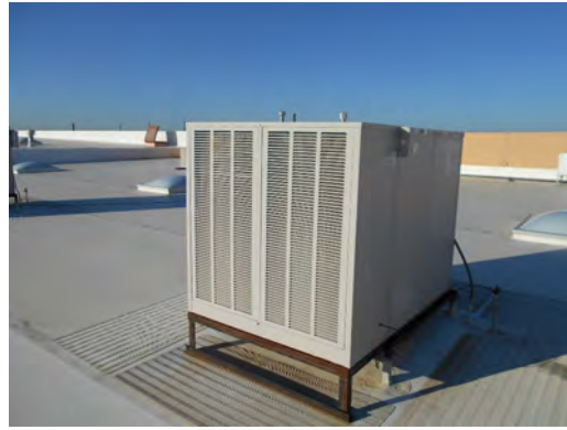
Canutillo_Central_Office Old evaporative coolers
