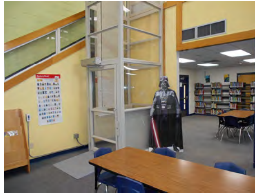
Canutillo_MS Library lift station is not ADA compliant
