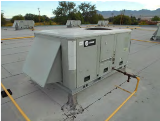
Damian_ES Roof top HVAC, old TRANE units
