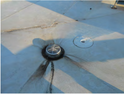
Childress ES_Roof drains require cleaning
