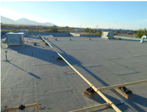
Childress ES_Roof mechanical equipment
