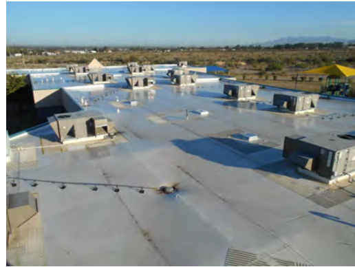
Childress ES_Roof mechanical equipment (2)
