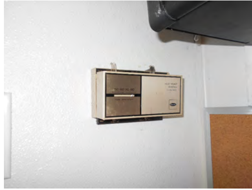
NW_Early_College_Campus Old HVAC controls
