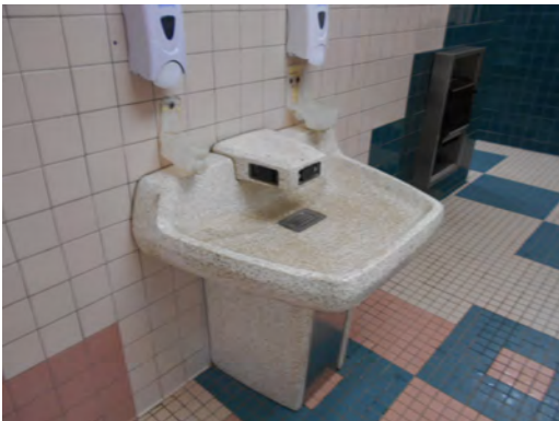
Childress ES_Restroom Lavatory
