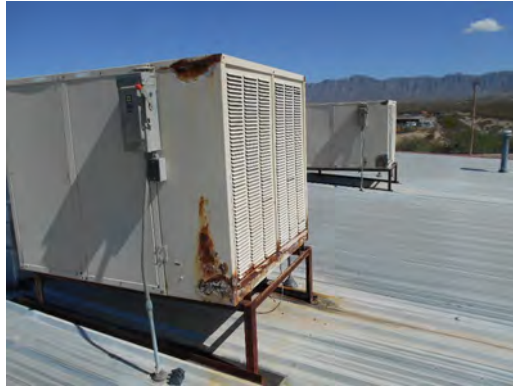
Canutillo_Facilities_Transportation Evaporative Cooler Deficiency
