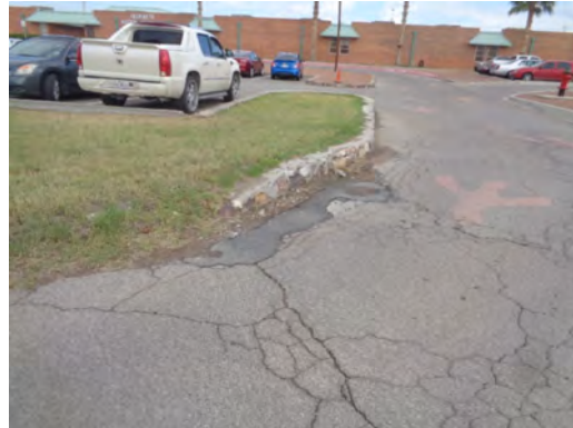
Alderete_MS Parking Lot / Roadways. Damage, replace and restripe
