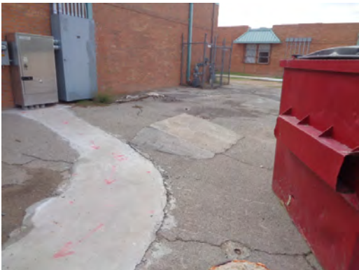
Alderete_MS Pavement, sidewalks cracked and missing
