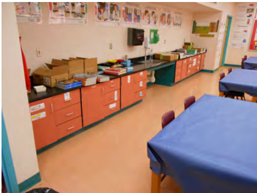
Childress ES_Base storage cabinets require replacement
