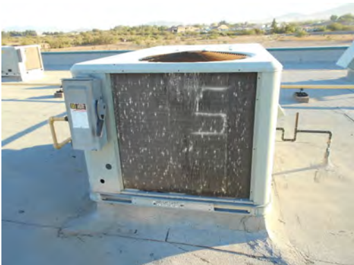
Childress ES_Roof Top Units require replacement
